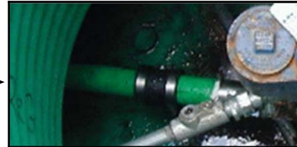
Closeup of Flexible Piping in a Sump
