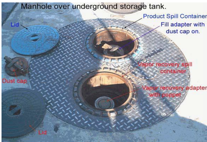
The image to the left shows the location of some Phase I Vapor Recovery System Components
