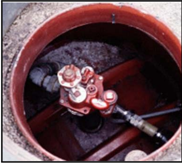
Sample STP Head in a Sump on Top of a Tank
