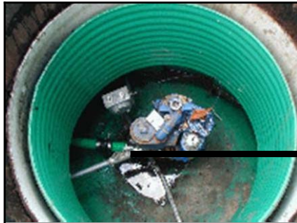
Sample Flexible Piping in a Sump
