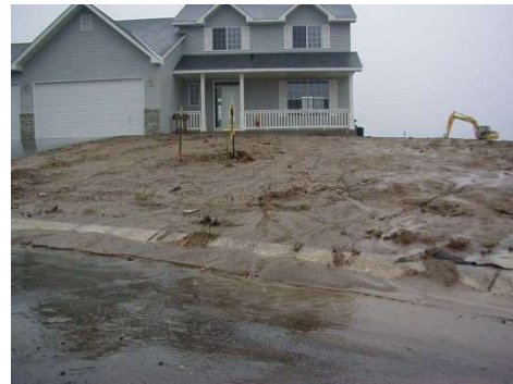
Example of erosion from a construction site.
