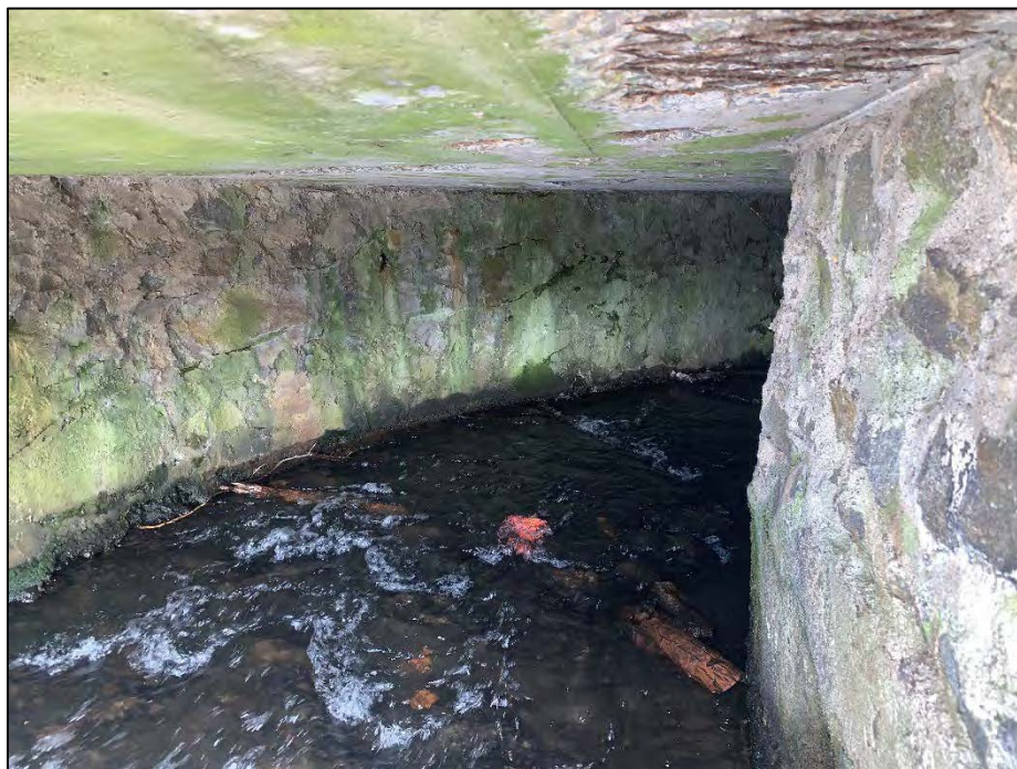
Photo No. 22.: Primary spillway culvert as viewed from the intake. Note the spalled areas along the ceiling with exposed reinforcement.
