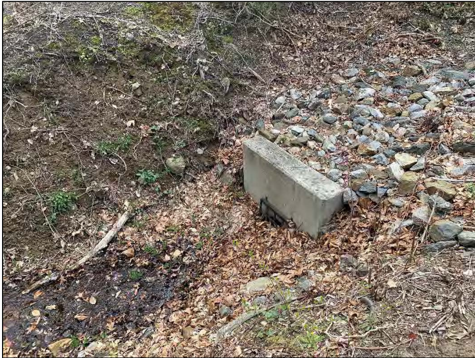
Photo No. 27.: Low level outlet discharge opening. Note buildup of leaves against opening.
