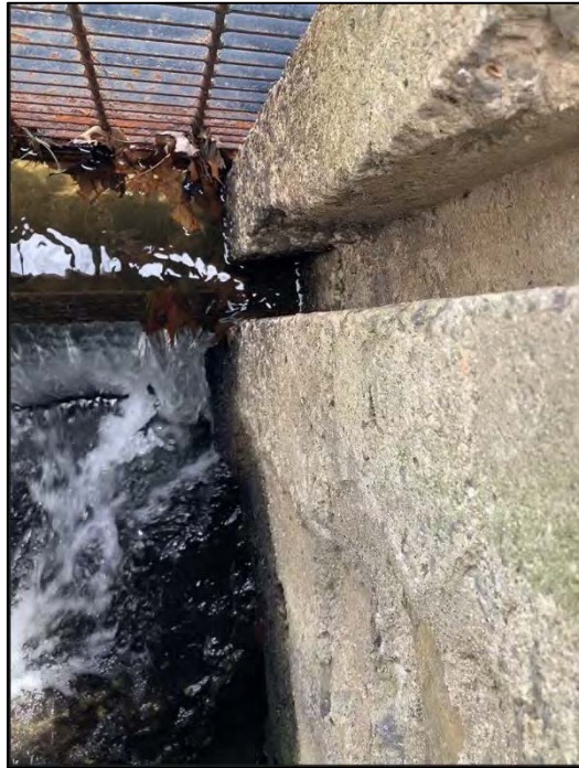
Photo No. 21.: Primary spillway stop log weir section right side looking down stop log slot. Note spalling within stop log slot and leakage under wall downstream of stop logs.
