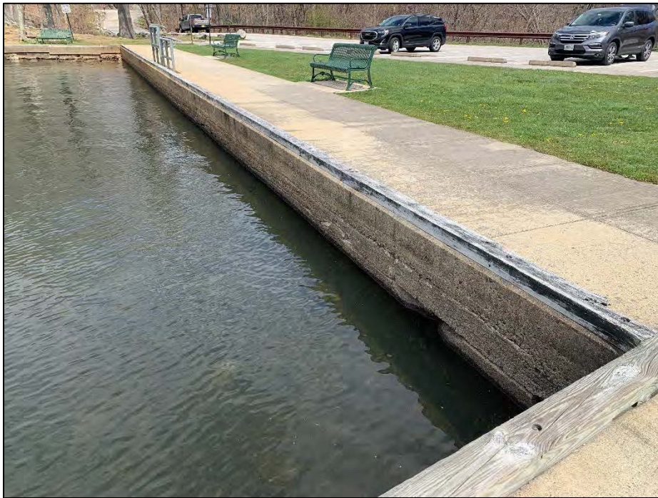
Photo No. 3.: Upstream side as viewed from low level outlet platform looking left. Note concrete spalling along waterline.
