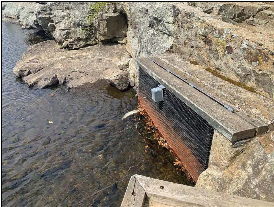
Photo No. 19.: Stop log-controlled primary spillway intake at the upstream side of the left abutment.
