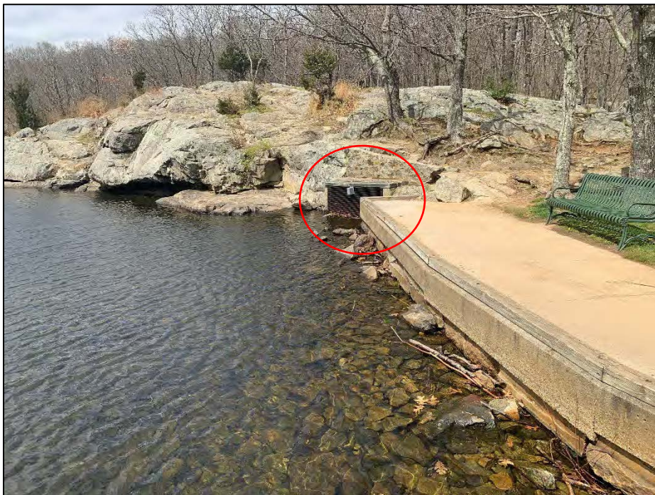
Photo No. 2.: Upstream side of dam as viewed from the bend near the left abutment looking left. Note the deteriorated and shifted concrete wall sections above the waterline. Circled is the primary spillway.
