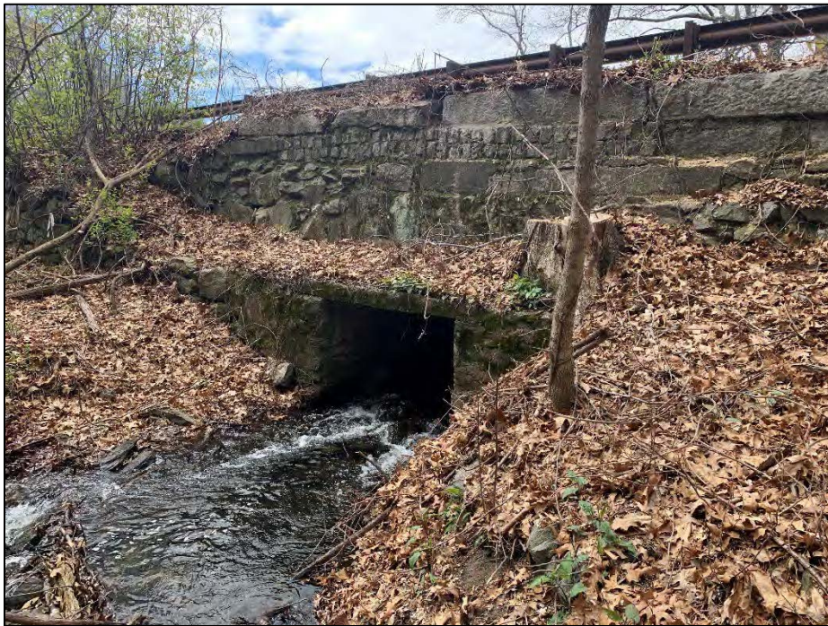
Photo No. 23.: Primary spillway discharge opening. Note tree trunk above the headwall.
