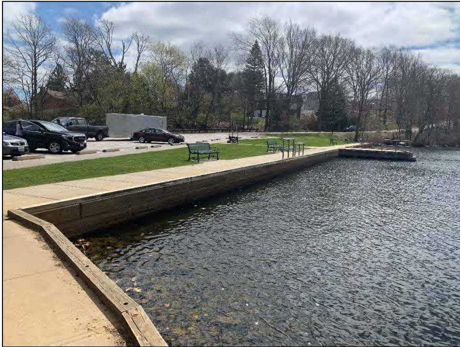
Photo No. 1.: Overview of the upstream side of the dam from the left abutment looking right.
