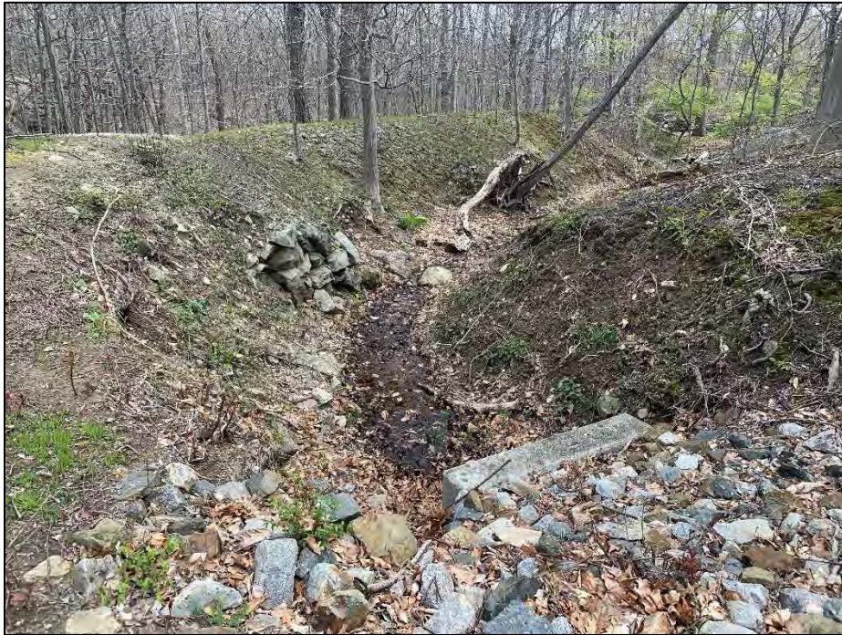
Photo No. 29.: Low level outlet discharge channel. Note deadfall cover within channel bottom.
