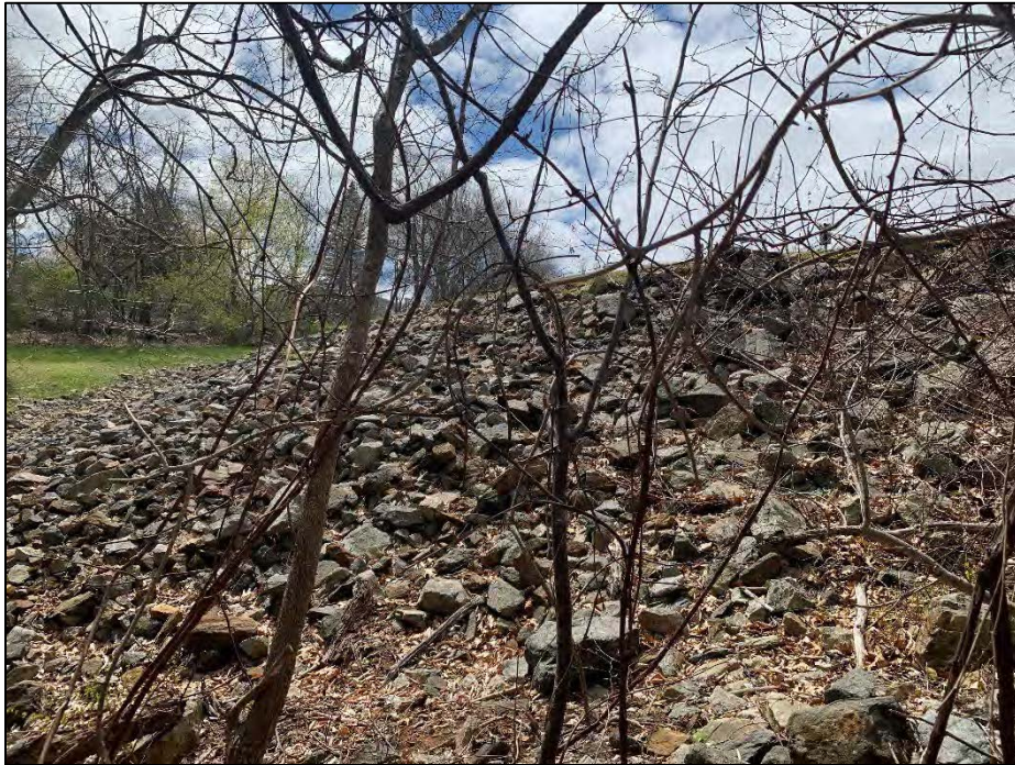
Photo No. 13.: Downstream slope as viewed from the primary spillway discharge looking right.
