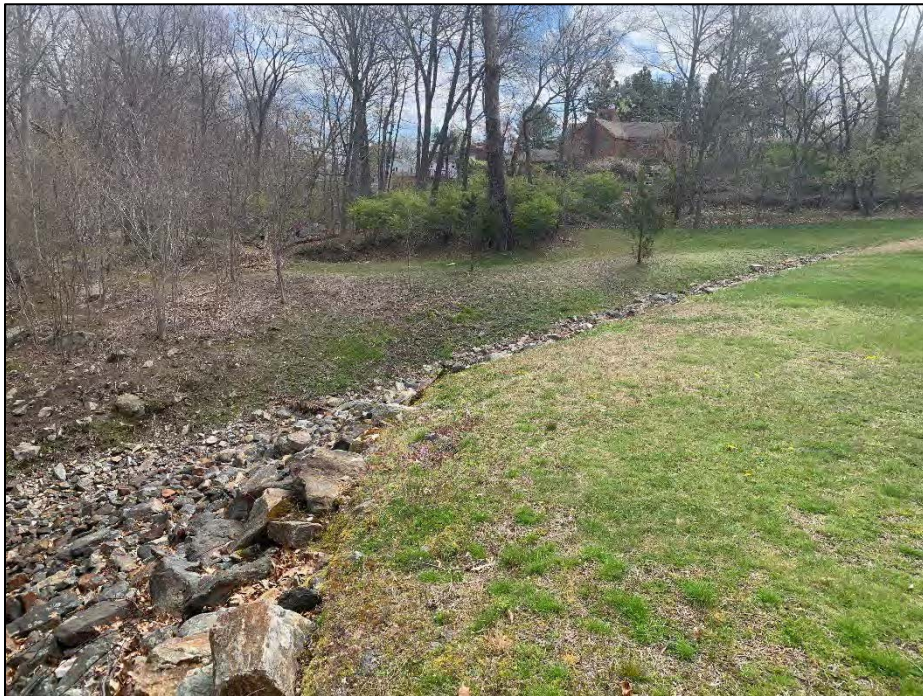
Photo No. 16.: Top of downstream slope as viewed from near Station 0+60 looking right.
