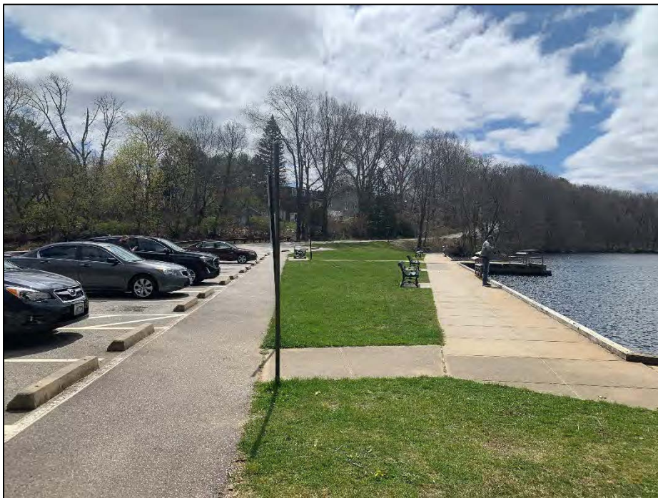
Photo No. 6.: Upstream side of crest looking right from near the end of the parking area.
