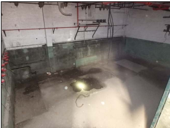
Photo 7 Overview of Room No. 2, located adjacent to the Turbine Room on September 9, 2018, as viewed from the east.
