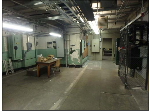
Photo 10 Overview of the northern portion of the main switchboard room located on the second floor on September 9, 2018, as viewed from the southeast.
