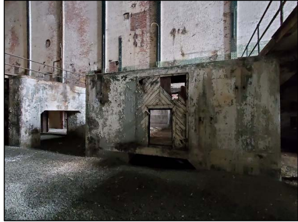
Photo 6 Concrete foundations associated with former turbines on September 2, 2021, as viewed from the southwest.
