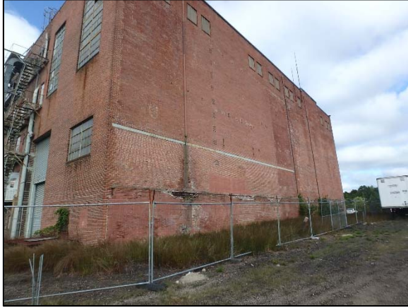
Photo 1 Overview of the east side of the Control House on September 9, 2018, as viewed from the southeast.
