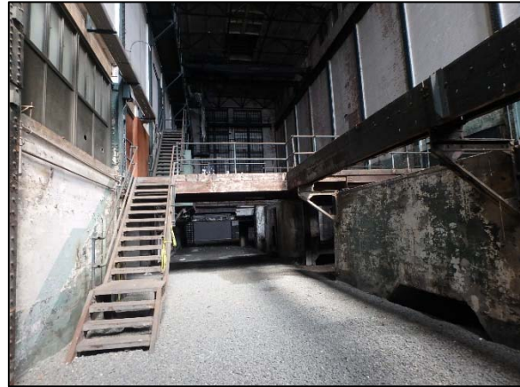
Photo 4 Overview of the Turbine Room on September 9, 2018, as viewed from the southeast. Note the trap rock covering the floor.
