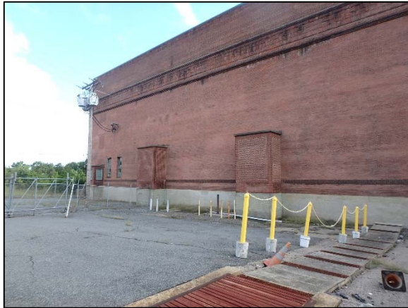
Photo 3 Overview of the west side of the Control House on September 9, 2018, as viewed from the southwest.
