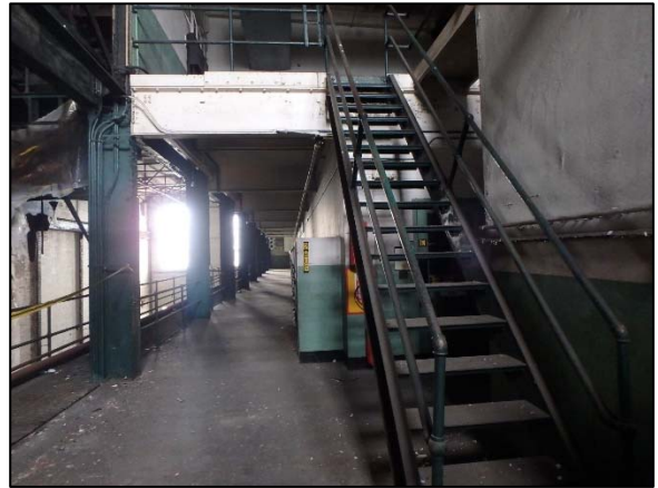
Photo 12 Overview of the mezzanine located on the fourth floor on September 9, 2018, as viewed from the north.
