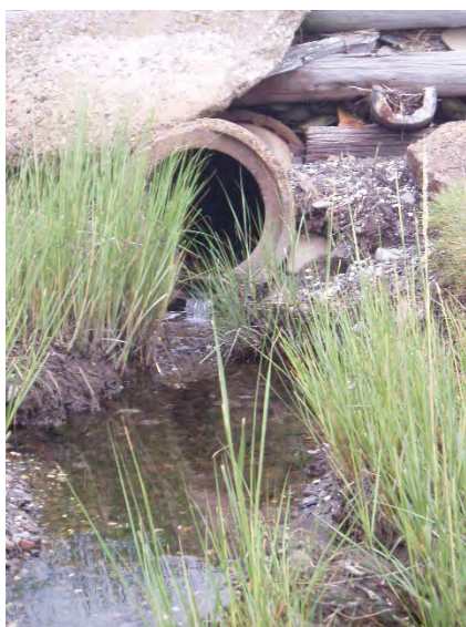
Figure 6: Source 3-300, a 48" concrete pipe draining an upland wetland on Prudence Island, just north of the T-Wharf.
