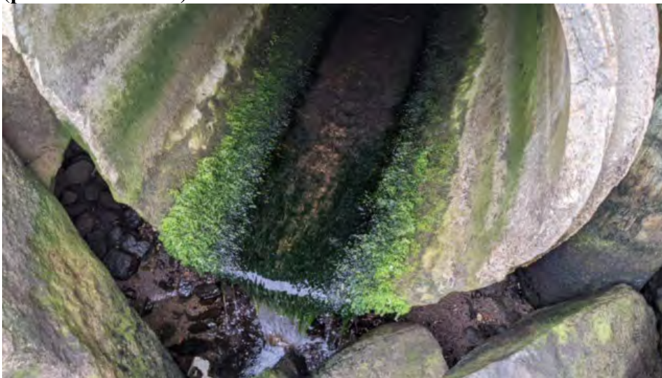
Figure 4: Source 2022-3-005, a 36" diameter pipe conveying stormwater to Bristol Harbor (prohibited waters).
