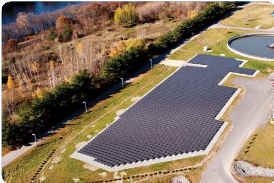
Greater Lawrence Sanitary District: 441-kW Solar PV Array (photo: Gregg Shupe)
