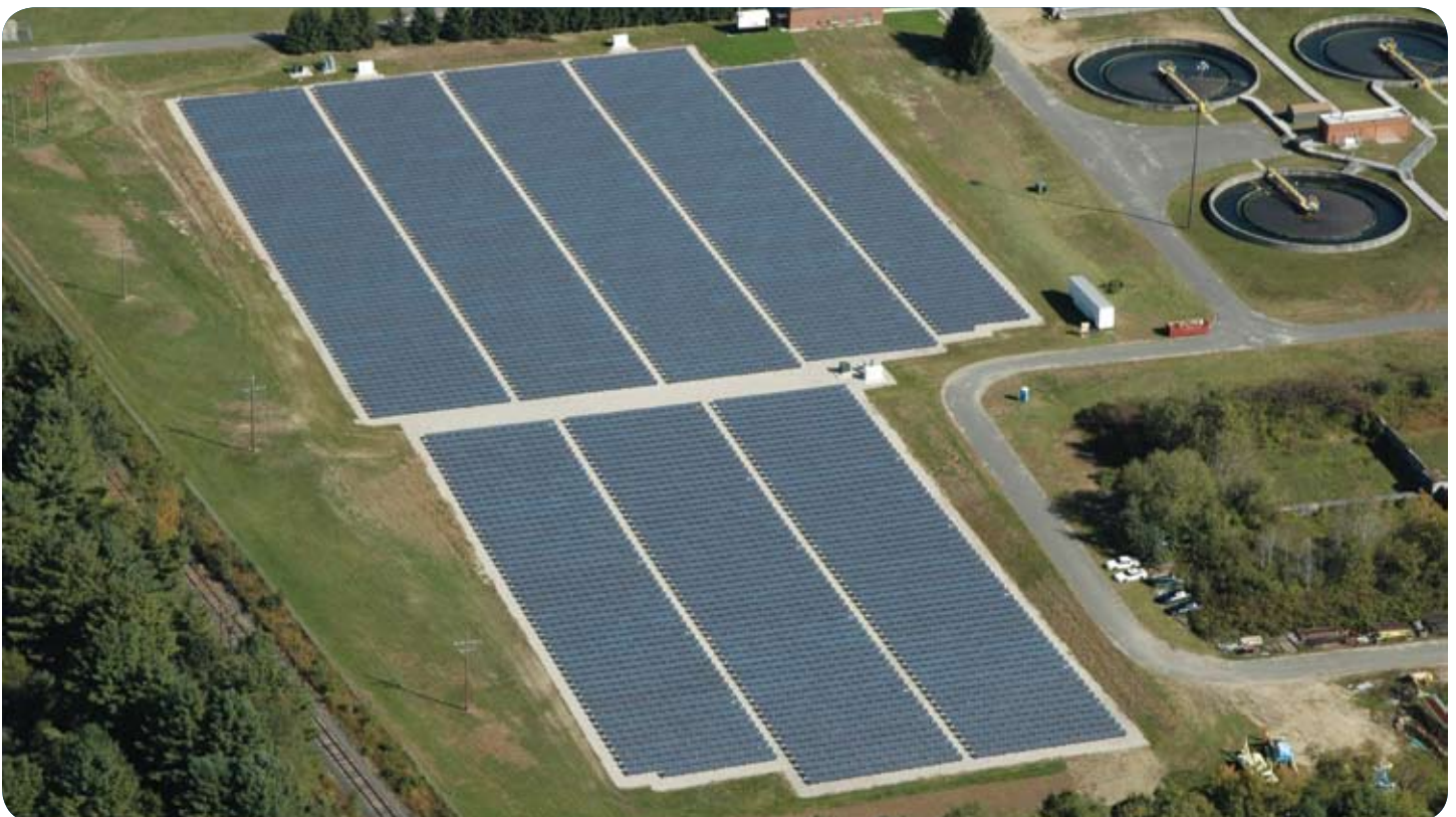
Pittsfield Wastewater Treatment Plant: 1.58-MW Solar PV Array (photo: Nexamp)
