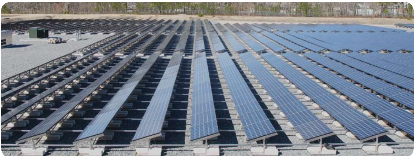
Barnstable Wastewater Treatment Facility: 819-kW Solar PV Array (photo: Nexamp)
