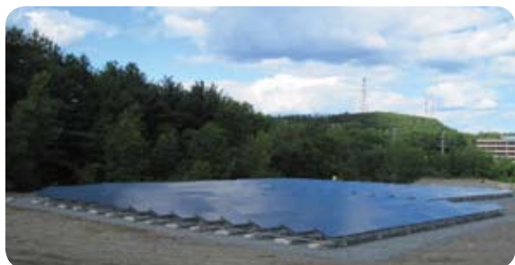
Boston Properties: 110-kW Solar PV Array (photo: Nexamp)
