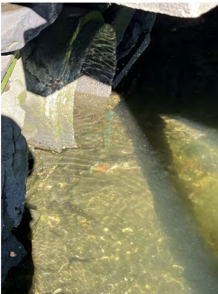
Figure 2: Source 8-2-213, 30" concrete pipe below Blu On The Water
