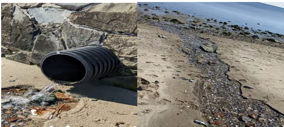
Figure 5: Source 1-008, an 18” corrugated plastic drain pipe draining storm water from the extension of Lippitt Ave in Warwick.
