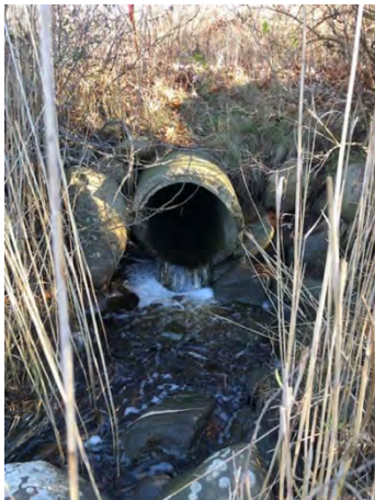
Figure 4: Source 2021-10-200 a small stream flowing through a culvert at Kenyon Farm, Narragansett, RI.
