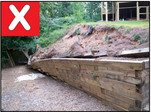
* Poorly engineered retaining wall.
