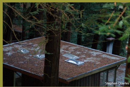
Photo 2. Minimal accumulation of vegetative debris accumulated on these dome-type skylights on this low-slope roof.
