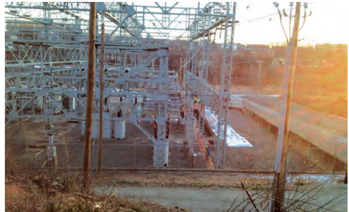
The majority of excavation associated with upgrading the existing Tidewater electrical substation is complete.
