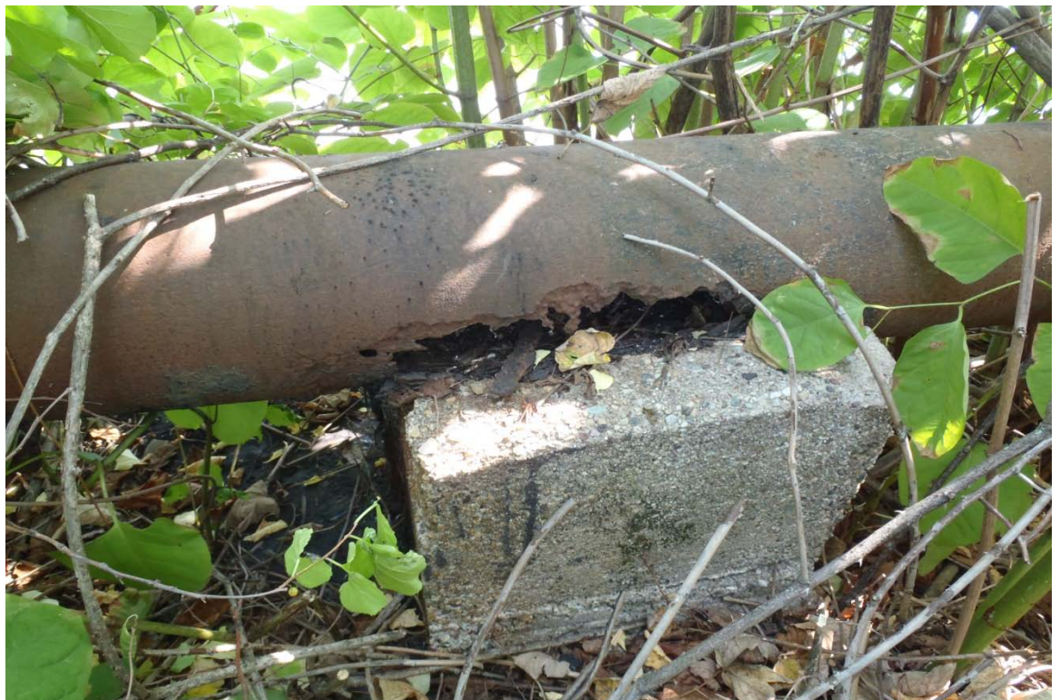
Photo 2: Broken pipe along riverbank. Pipe leak of apparent coal tar-like material.
