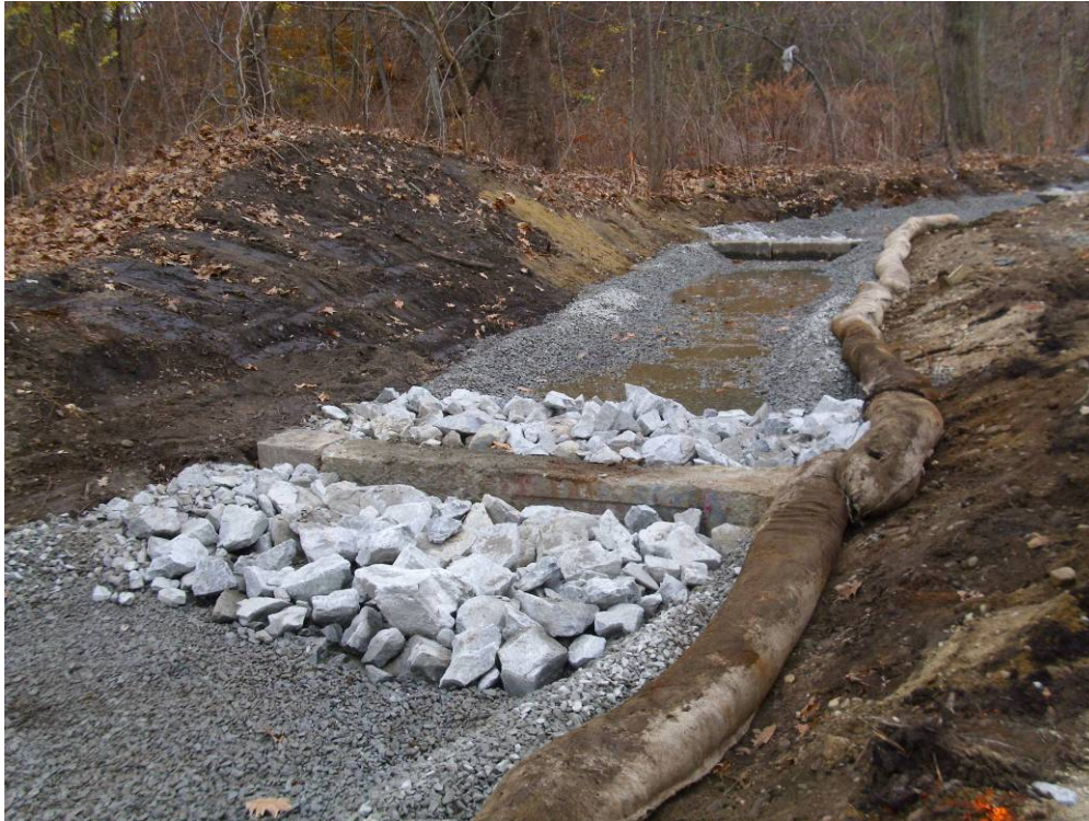
Photograph No. 15 Installation of check-dams in the downstream portion of the sluiceway (11/15/10).
