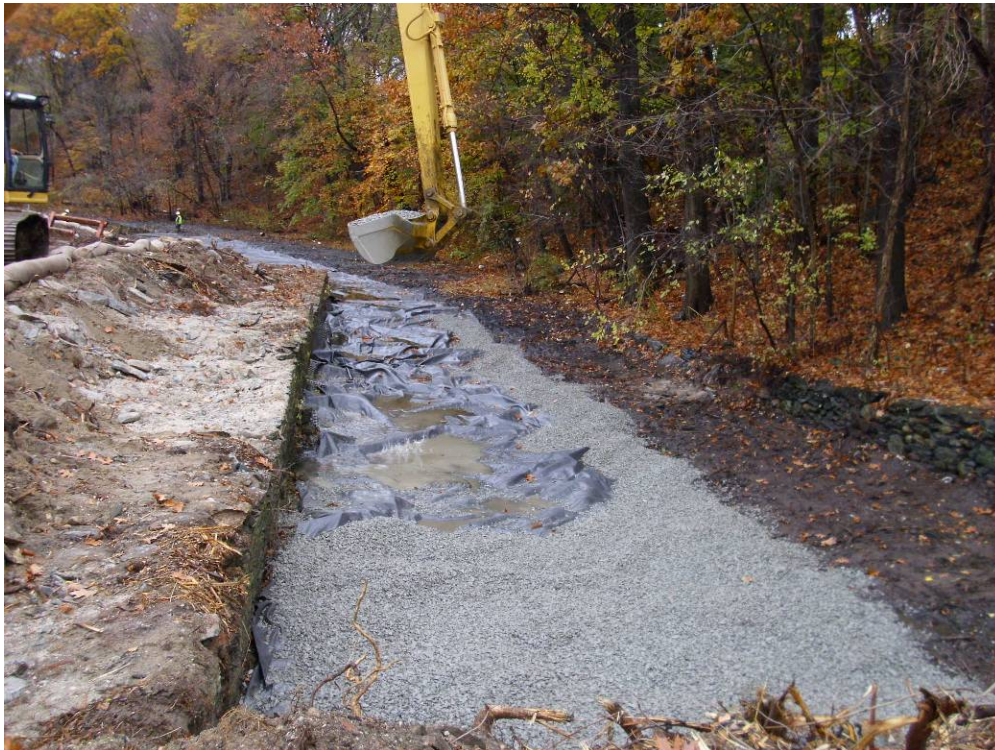
Photograph No. 8 Installation of crushed stone over the geotextile in the sluiceway (11/5/10).
