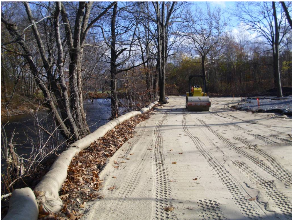
Photograph No. 16 Installation of fill material over geotextile in the northern portion of the site (11/17/10).
