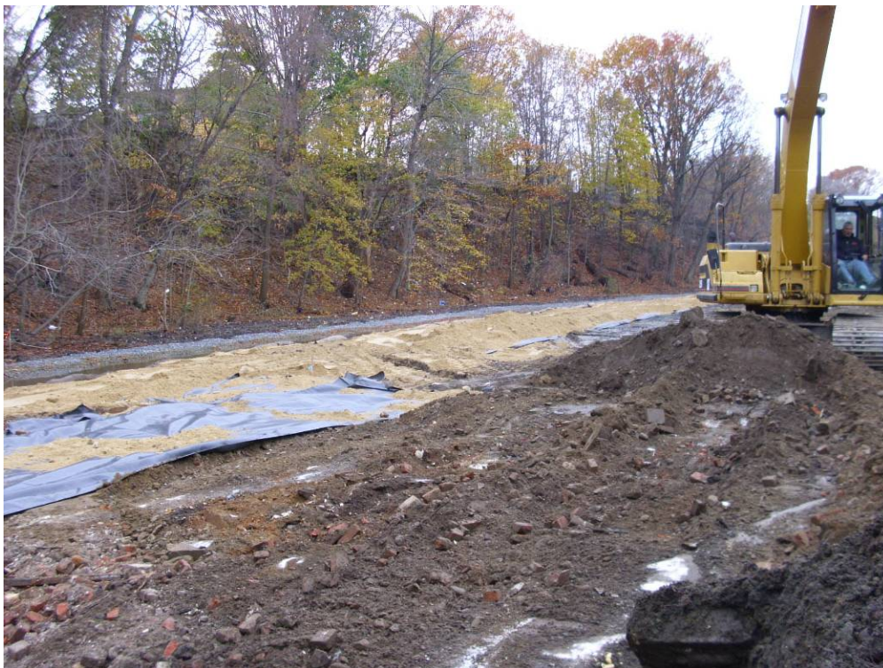
Photograph No. 12 Installation of fill material over geotextile in the southern portion of the site (11/10/10).
