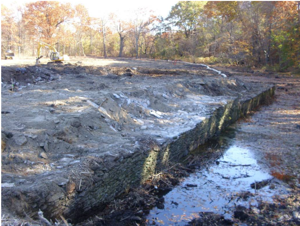
Photograph No. 6 Clearing the site adjacent to the sluiceway in the southern portion of the site (11/3/10).
