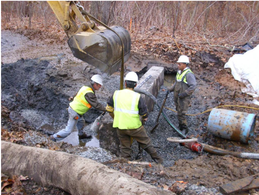
Photograph No. 14 Installation of stone check-dams in the downstream portion of the sluiceway (11/10/10).
