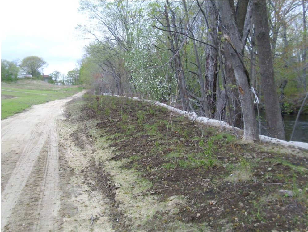
Photograph No. 29 Plantings in the northern portion of the site along the Woonasquatucket River (5/5/11).
