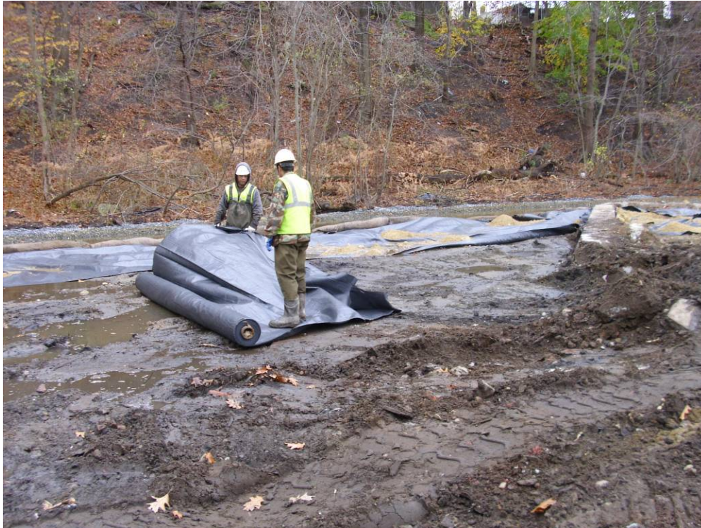
Photograph No. 11 Installation of geotextile fabric in the southern portion of the site (11/10/10).
