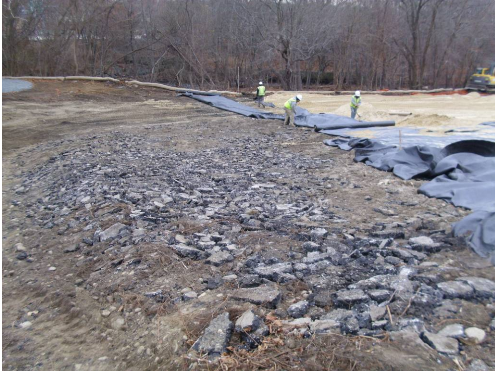
Photograph No. 23 Installation of geotextile in the western-central portion of the site (12/3/10).
