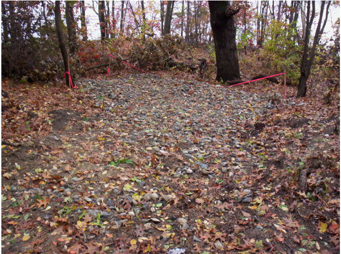
1631. Rip rap placed at the hot spot excavation at the southwest swale, looking south
