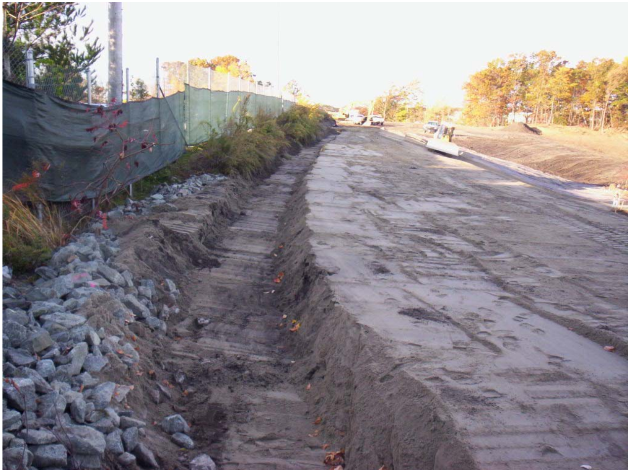
1577. Looking southwest at installed anchor trench at the top of slope at Area 4. Dozer is fine grading buffer sand.
