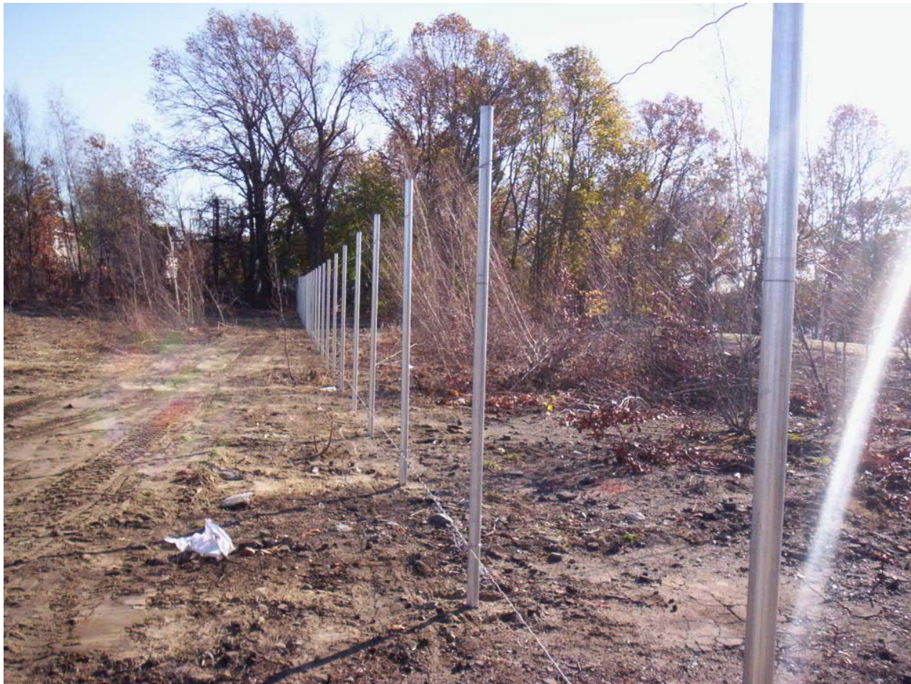
1685. Fence posts installed east of area 1at the boundary with Parcel C, looking southeast
