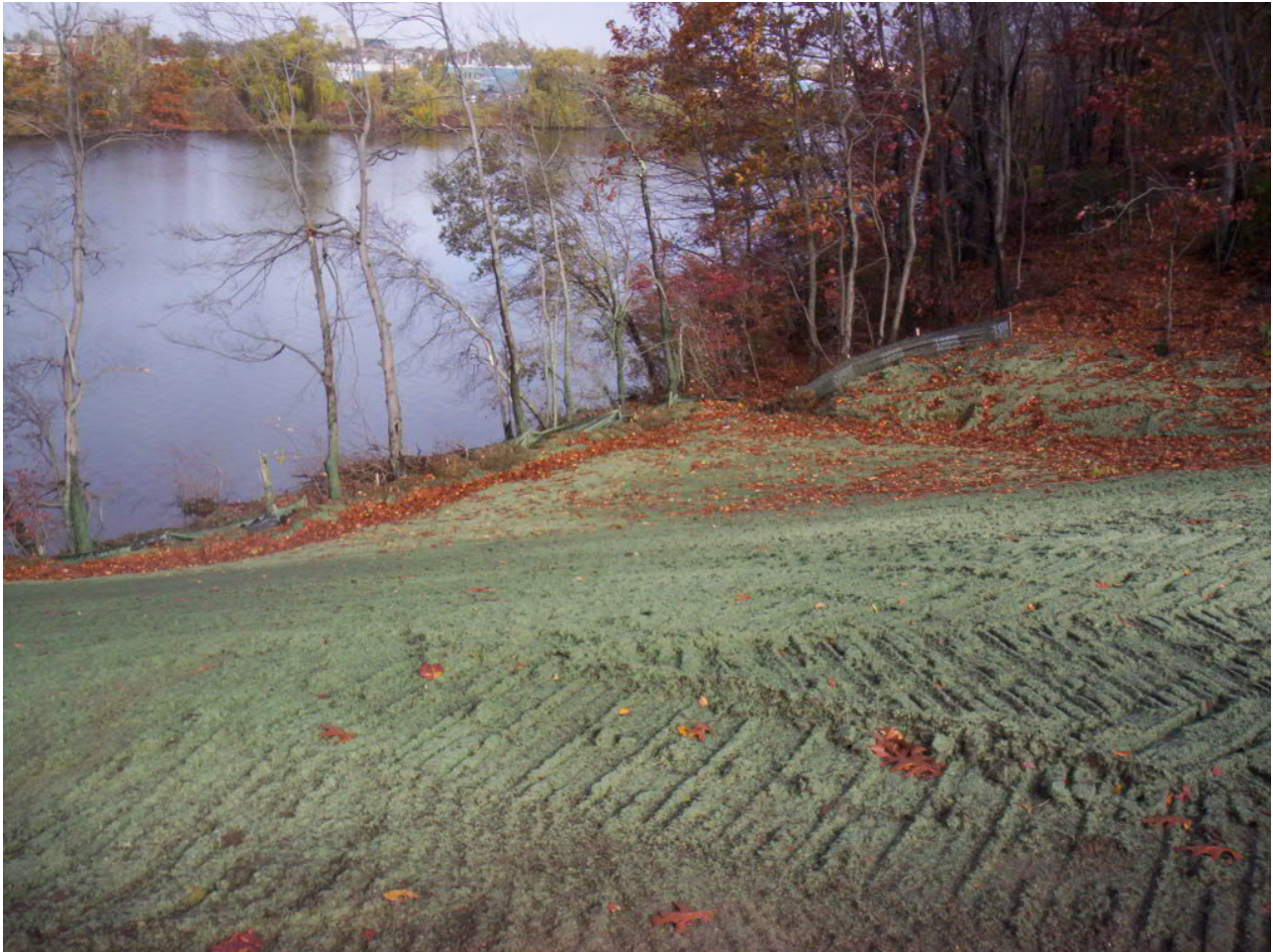
1623. Topsoil and hydroseeding remained in good condition after the hurricane at Area 2, looking northwest
