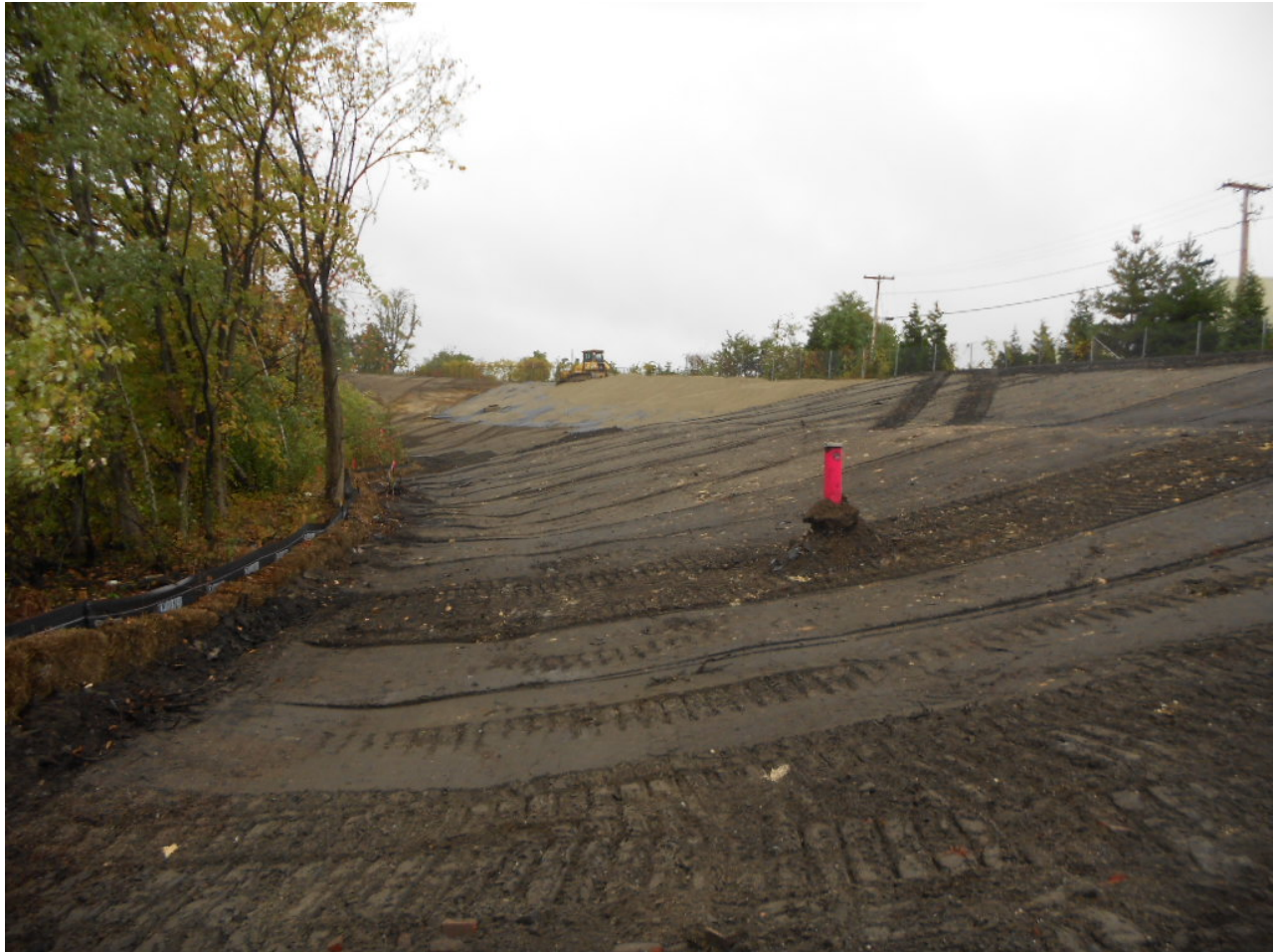
1034. Dozer placing cover soil on geotextile at Area 5, upland cap, looking northeast
