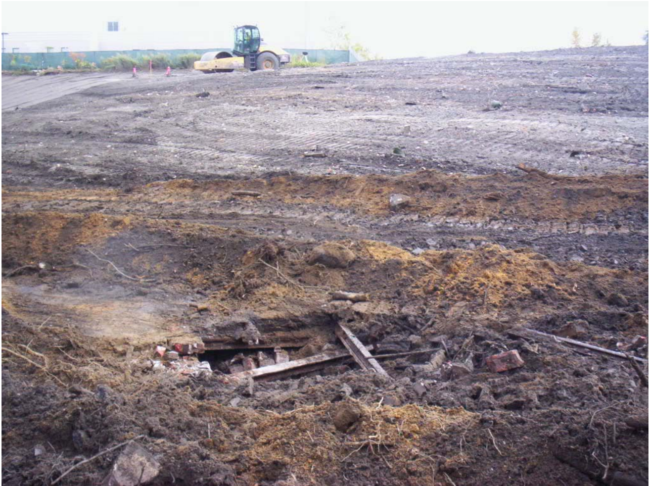
1054. Brick structure uncovered near the toe of slope at Area 3 during sub-grading, looking southeast
