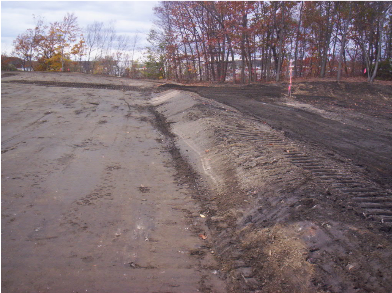
1659. Opening in berm created for gate, looking west. Roller compacted laydown area.
