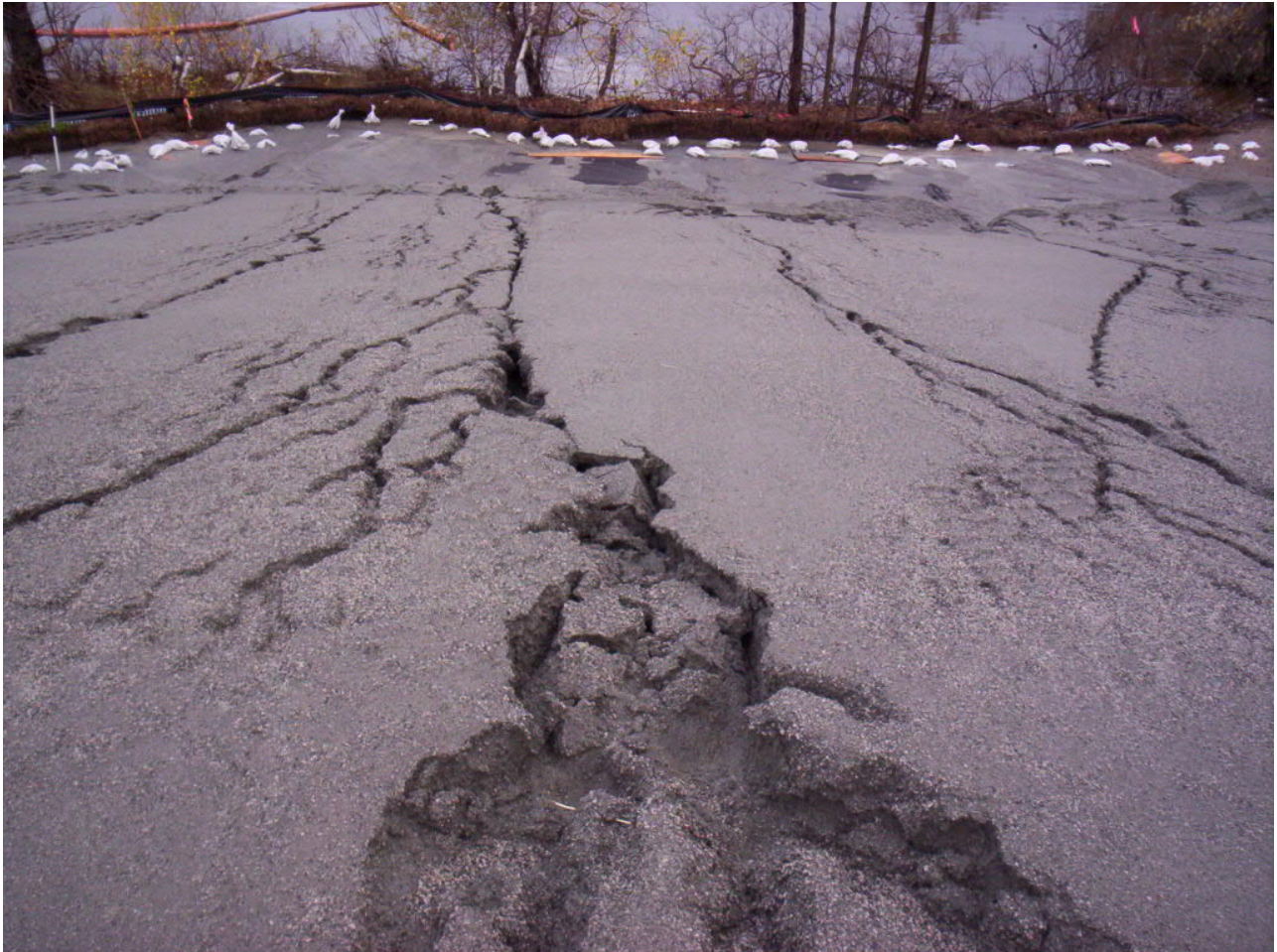
1628. Erosion at the Area 4 slope due to overnight rain event, looking north
