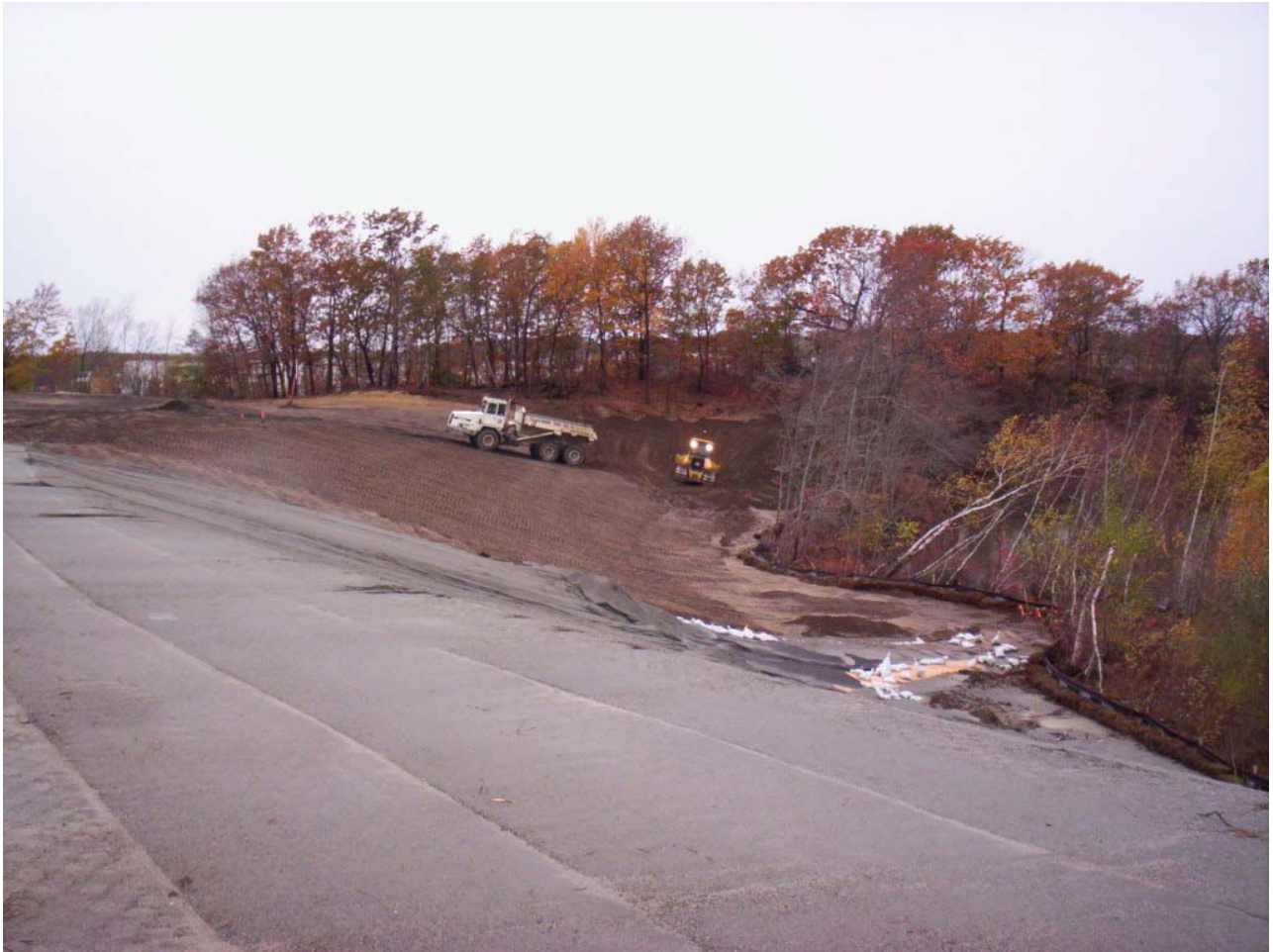
1629. Placing topsoil for the wetland buffer cap at the western side of Area 3, looking west.
