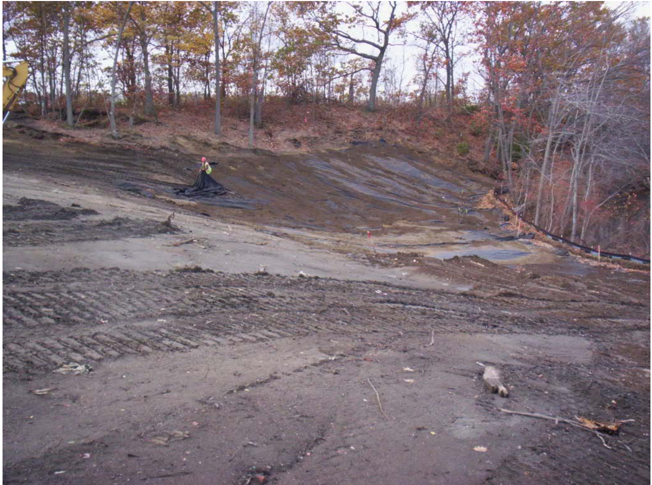
1627. Geotextile and topsoil placement at the western side of Area 3, looking west
