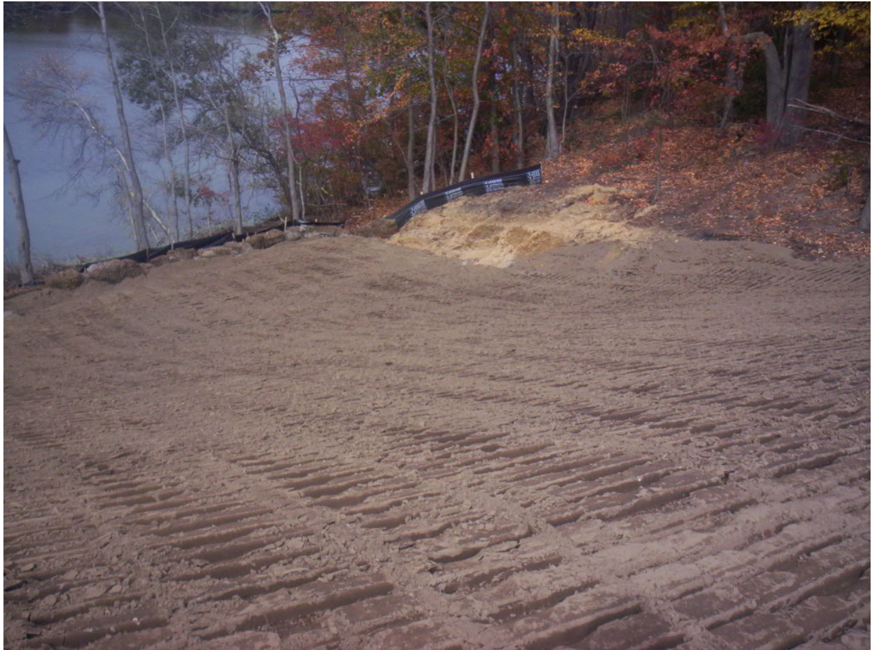
1594. Looking northwest at topsoil placed at Area 2 following repair of eroded cover soil
