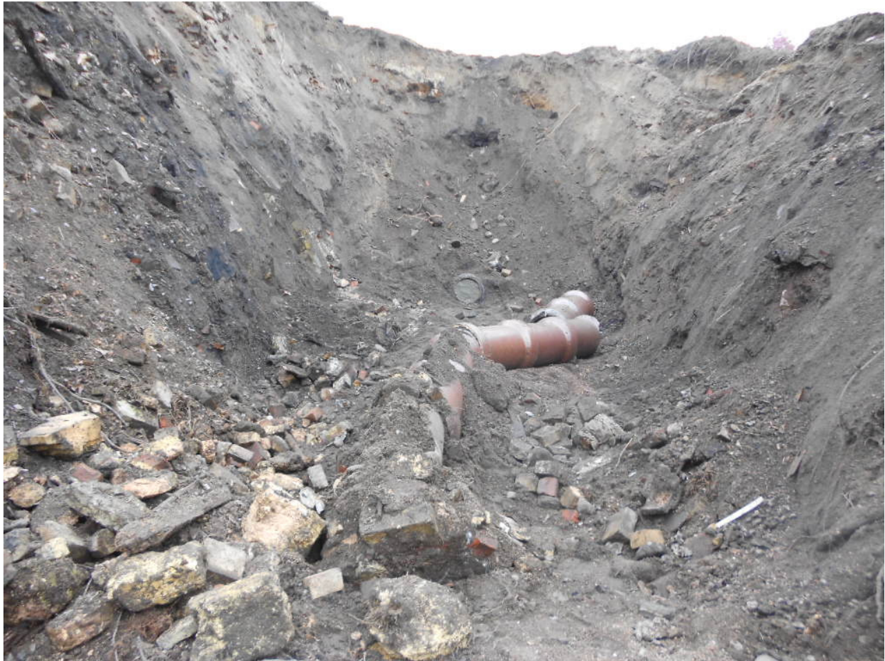
1000. Storm drain pipe plugged under the pile of industrial fill in Area 5, looking east toward HS parking lot
