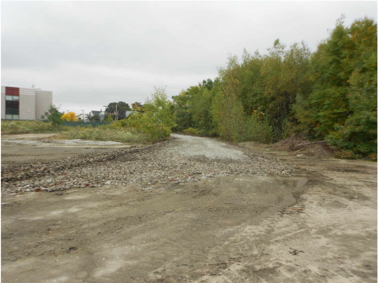
1010. Construction entrance extended with rip rap material from former slag area, looking east
