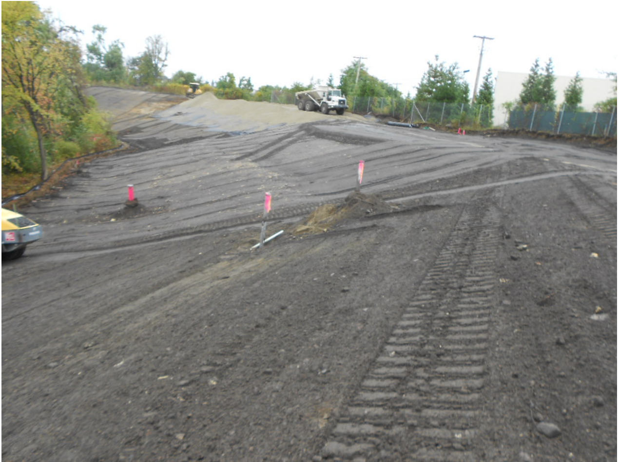
1037. Dozer placing cover soil on geotextile at Area 5, upland cap, looking northeast
