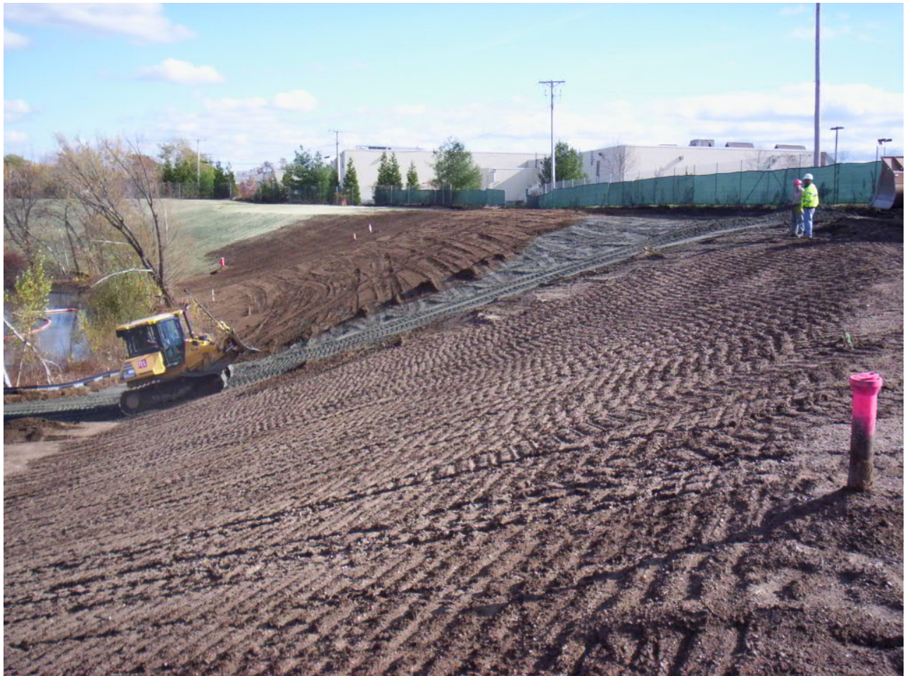
1634. Dozer placing topsoil on top of protective soil at Area 4, looking east
