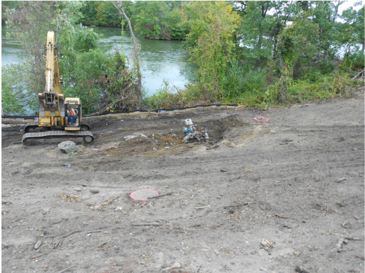
0917. Pump and piping for the former pump house at the northeast of the site, looking northwest
