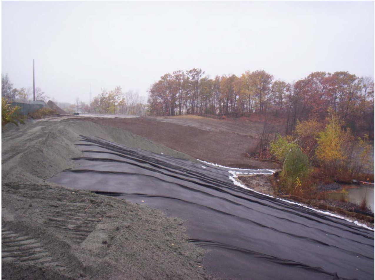
1614. Protective soil placed at the edges of the drainage geocomposite at Area 4 during the hurricane, looking southwest
