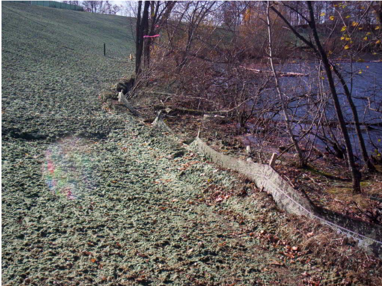
1681. Toe of slope at Area 5 after Nor'easter, looking southwest
