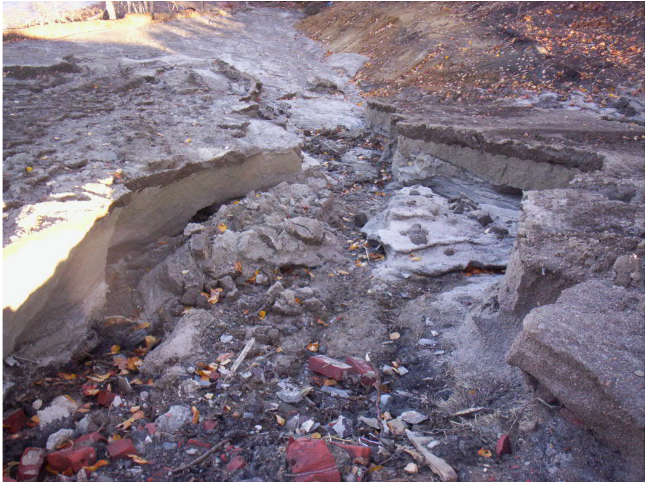
1573. Cover soil and topsoil eroded at Area 2 due to the rain event during the weekend of 10/20/12 and 10/21/12, looking west
