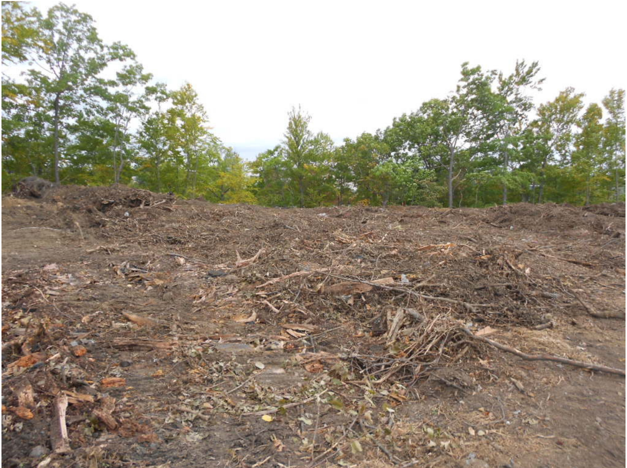
0964. Material remaining after stumps were sheared and chipped near Area 2, looking southwest
