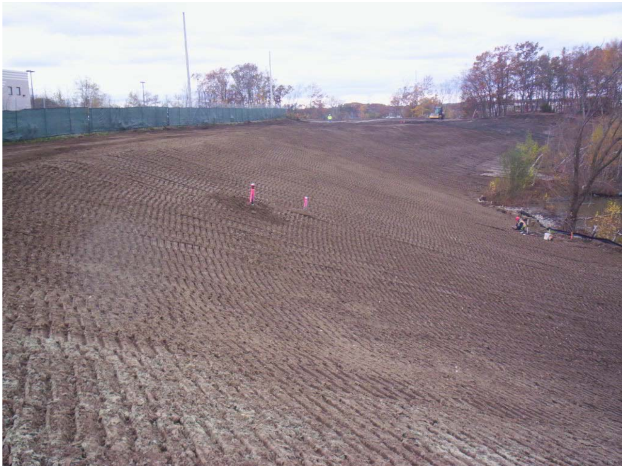
1651. Looking southwest at Areas 3 and 4. Final grading achieved. Raising MW-231 (S, D, or probe – not confirmed) at center right of photo
