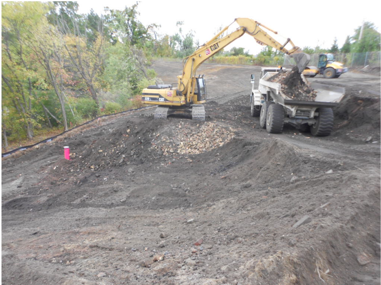
1024. Regrading industrial fill at Area 5 with excavator and off-road dump and compacting Area 5 sub-grade with roller, looking northeast
