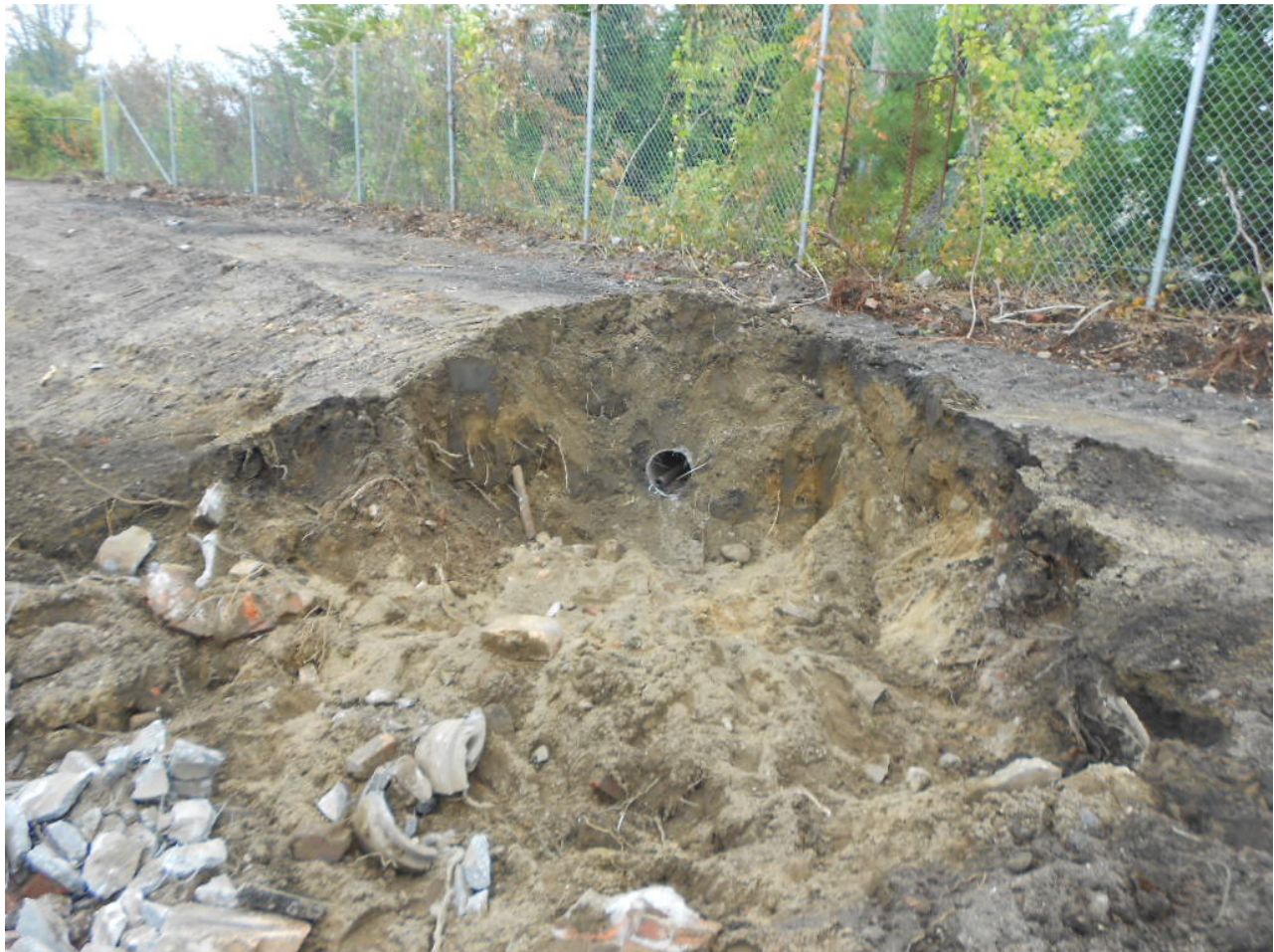
1001. Storm drain to be plugged at the top of the bank in Area 5, looking east
