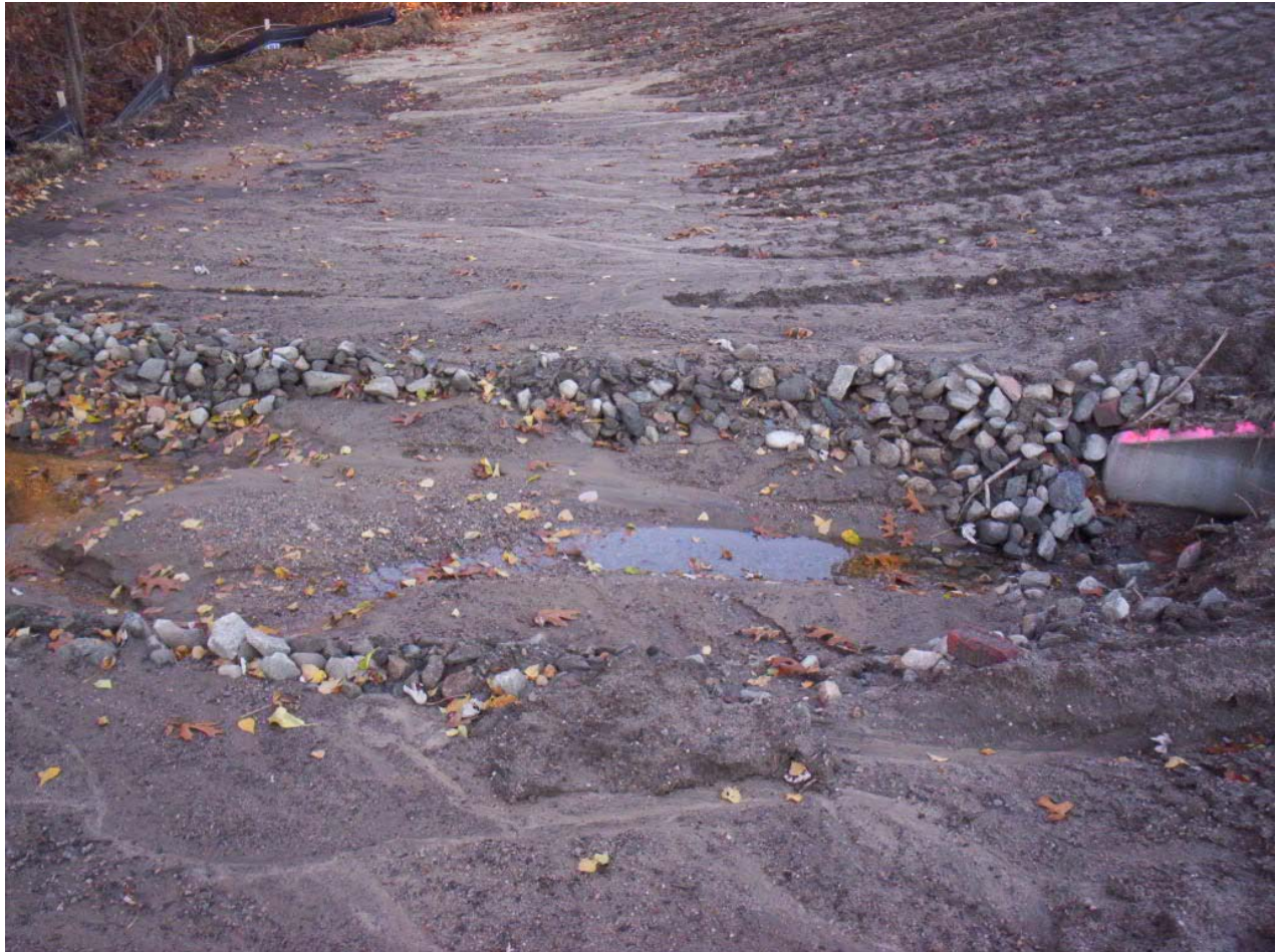
1570. Rip rap at storm drain outlet filled with sediment from recently placed topsoil at Area 5 due to the rain event during the weekend of 10/20/12 and 10/21/12, looking north
