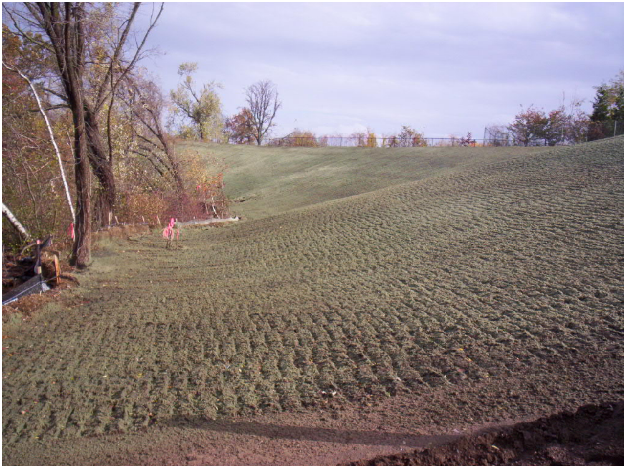
1620. Topsoil and hydroseeding remained in good condition after the hurricane at Area 5, looking northeast from the toe of slope
