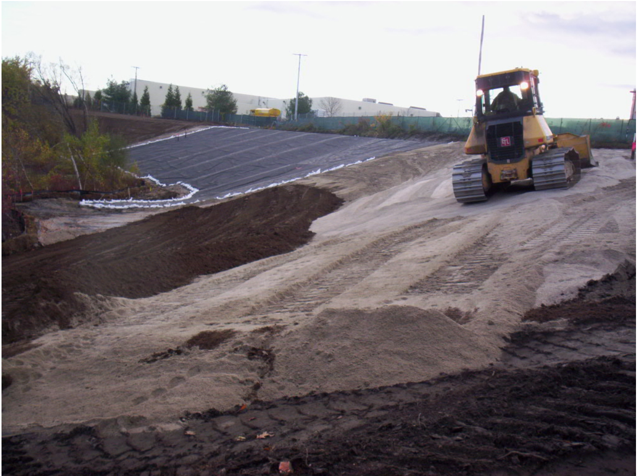
1599. Dozer placing cover soil at the upland soil cap at Area 3, looking east
