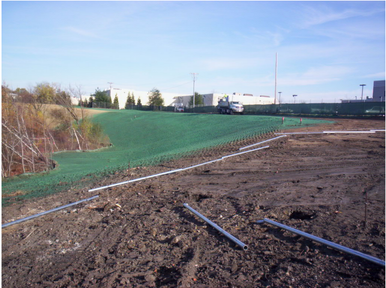
1667. Areas 3 and 4 hydroseeded, looking east. Posts set out for fence installation in the foreground.
