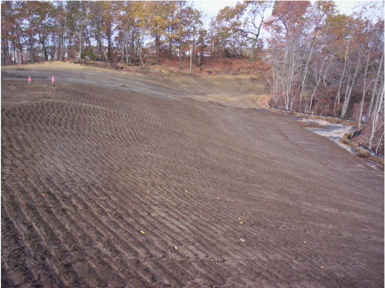
1621. Topsoil remained in good condition after the hurricane at Area 3, looking west
