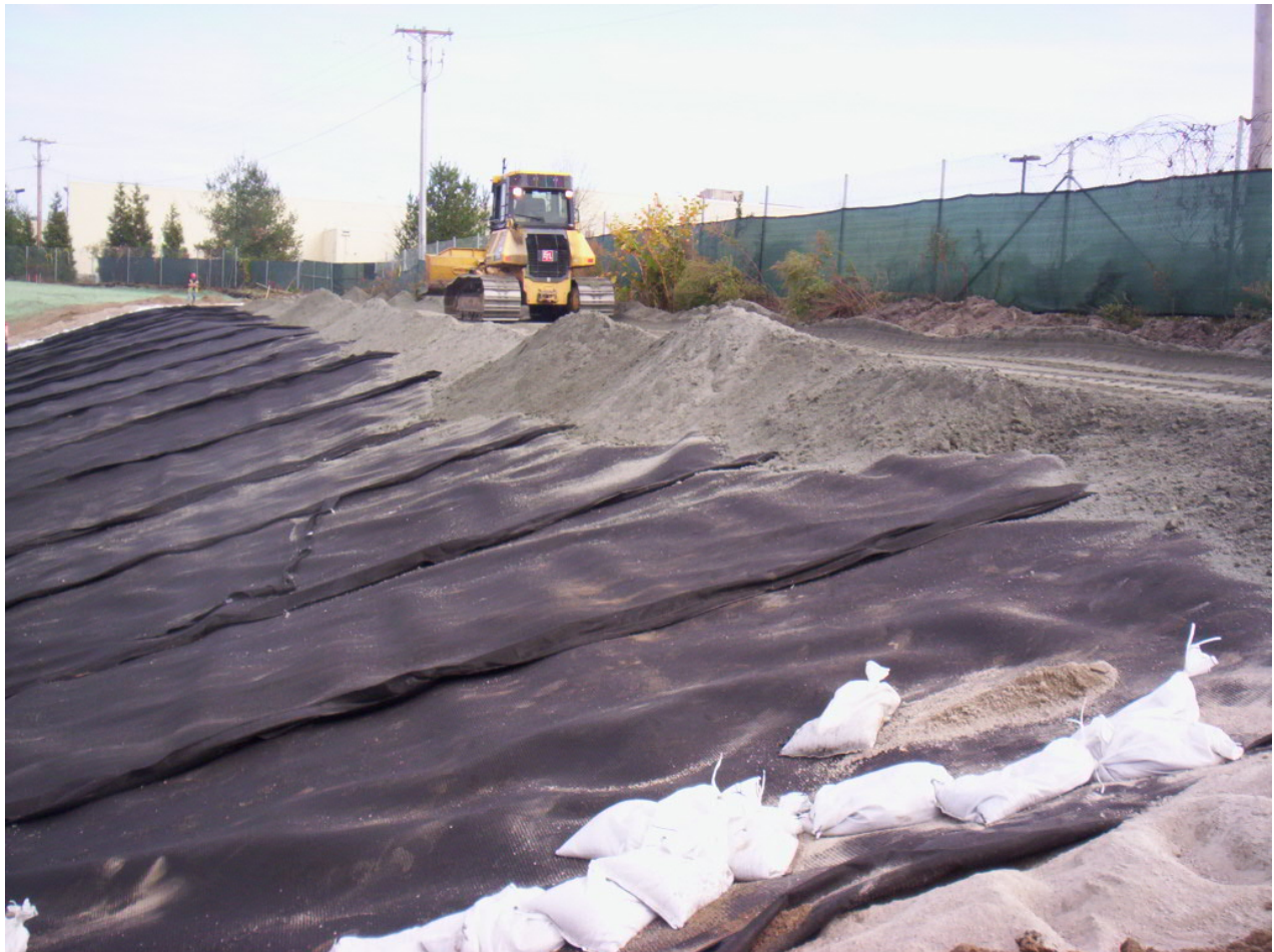
1612. Protective soil backfilled at anchor trench and at top of slope at Area 4, looking east
