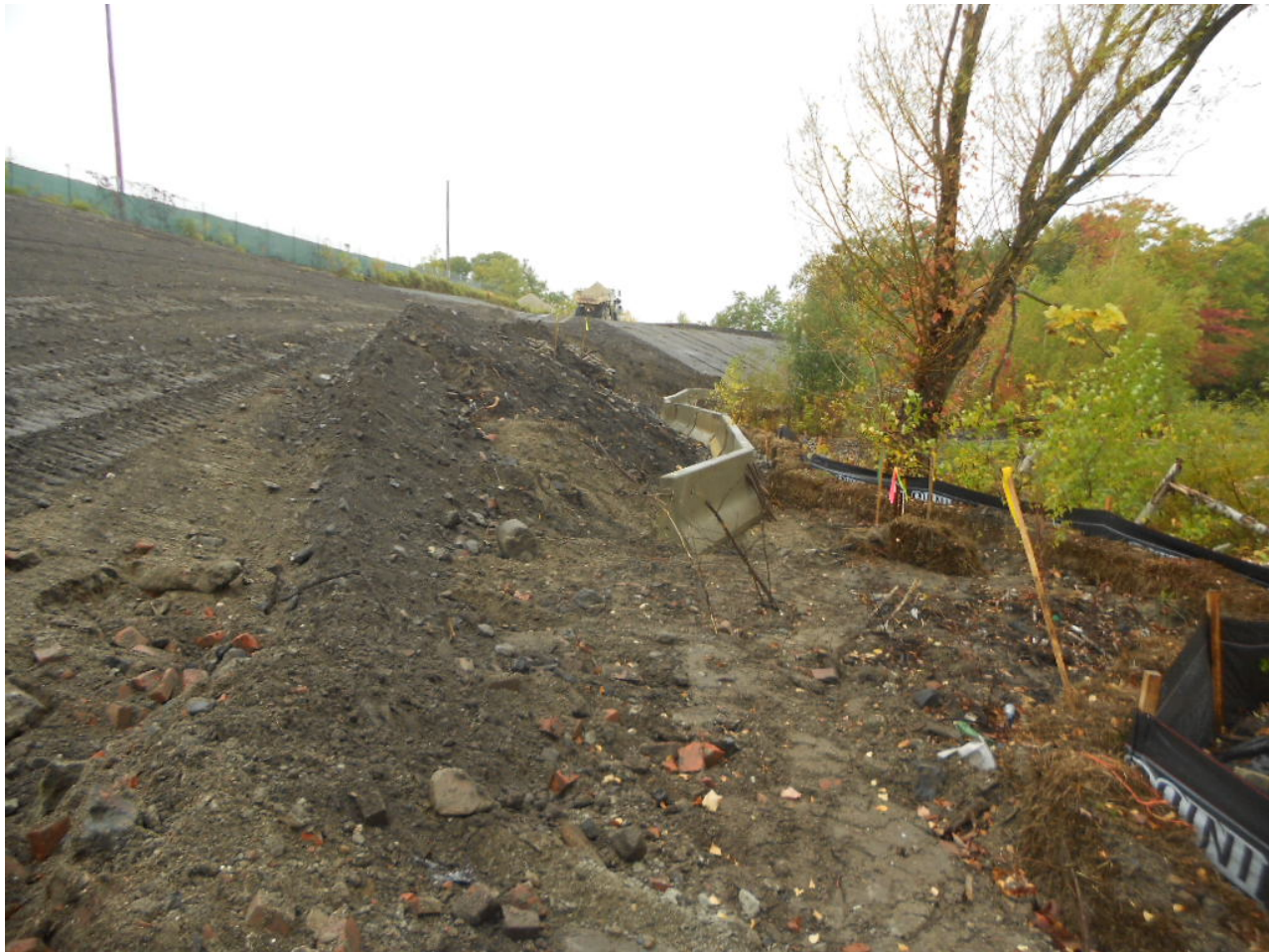
1033. Jersey Barrier retaining wall installed at the toe of slope at Area 4, looking southwest
