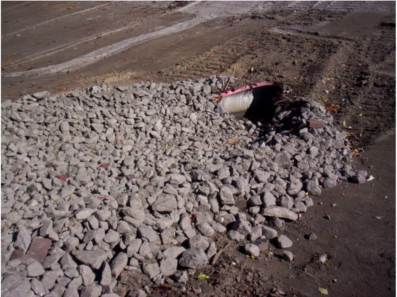
1555. Rip rap placed at the storm drain (from the detention basin) outlet
