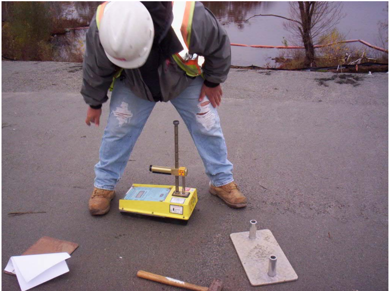
1630. Compaction testing on the protective soil at the top of the slope at Area 4
