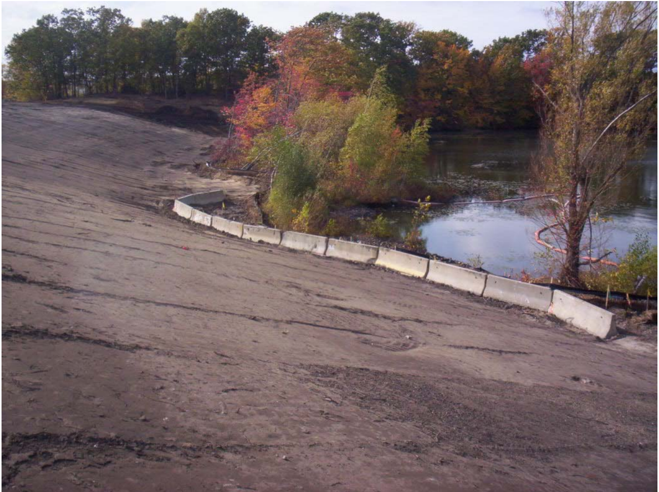
1056. Looking west at sub-grade preparation and Jersey Barrier retaining wall at Area 3 and Area 4
