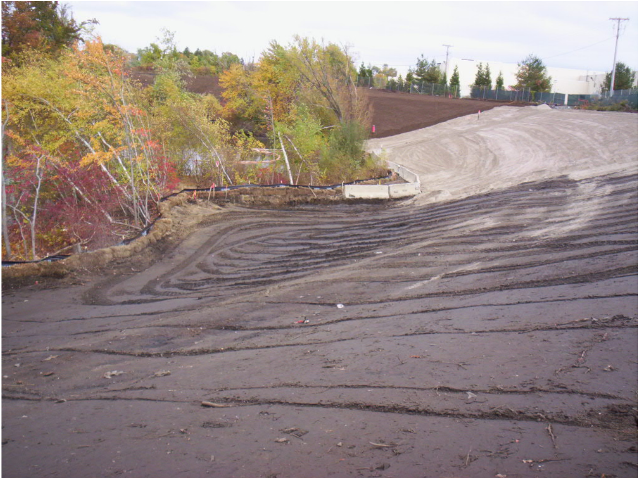
1567. Looking east from Area 3 at the finished grade at Area 5 and buffer sand at Area 4
