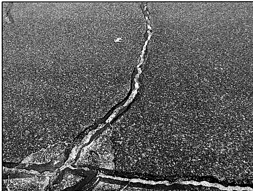
Photo 18: Example of cracking and previous fill efforts (see Photo Location Figure)
