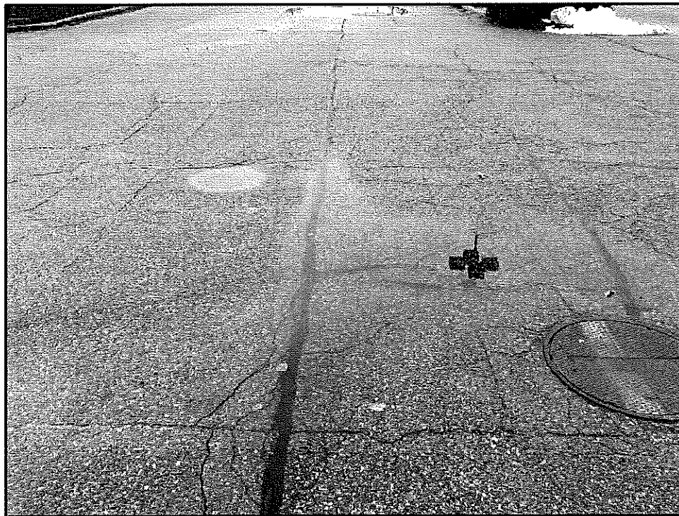
Photo 15: Puddling (see Photo Location Figure)
