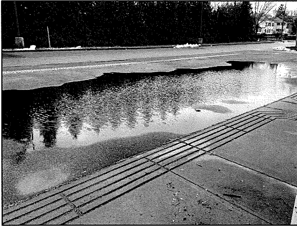
Photo 24: Puddling (see Photo Location Figure)
