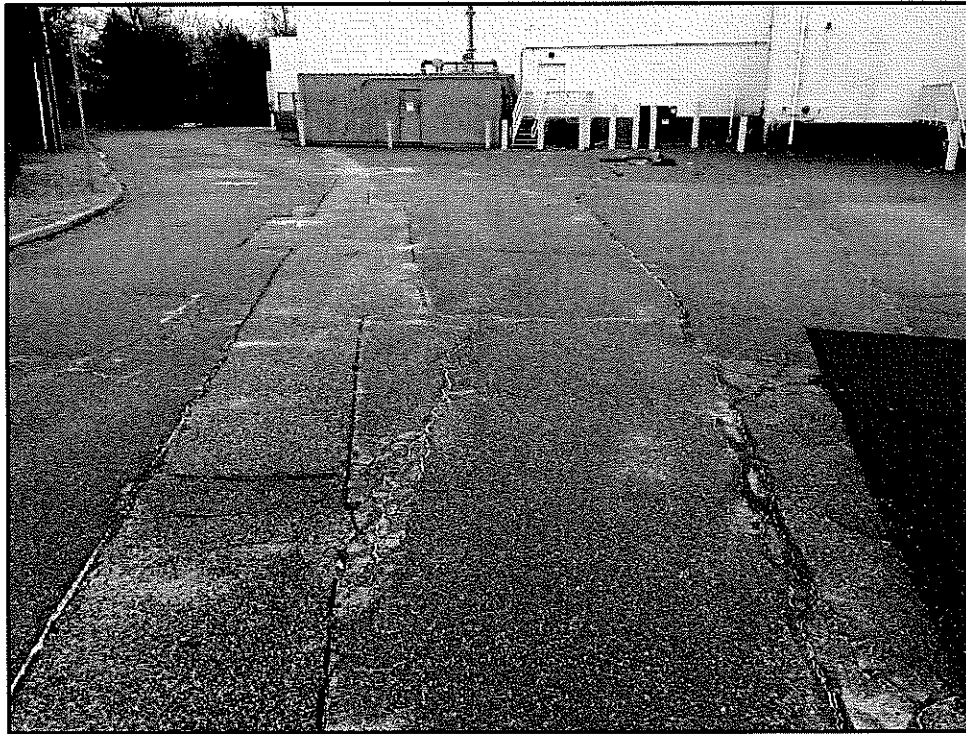
Photo 30: Pavement cracking (see Photo Location Figure)
