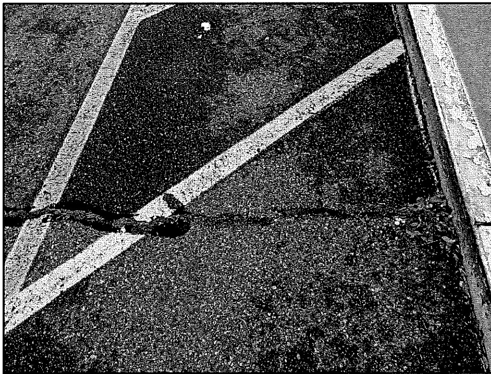
Photo 3: Example of cracking and previous fill efforts (see Photo Location Figure)
