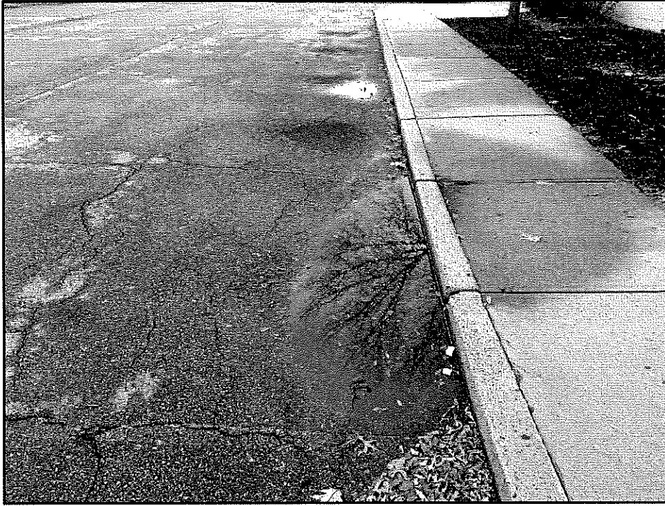
Photo 36: Puddling (see Photo Location Figure)
