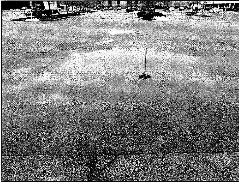
Photo 14: Puddling (see Photo Location Figure)
