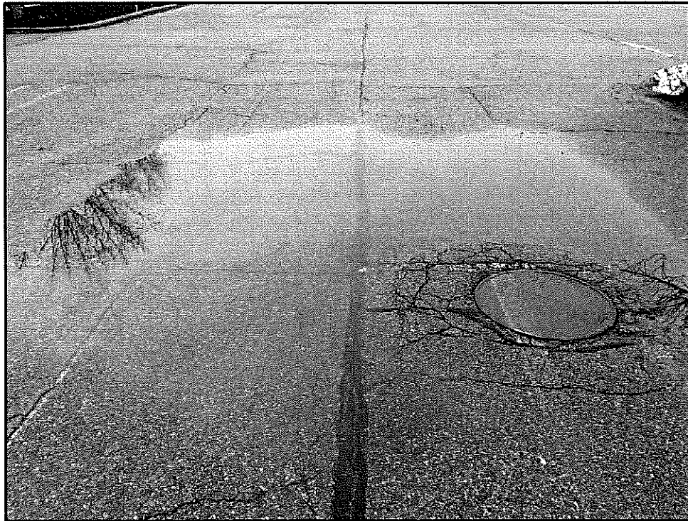
Photo 16: Puddling (see Photo Location Figure)
