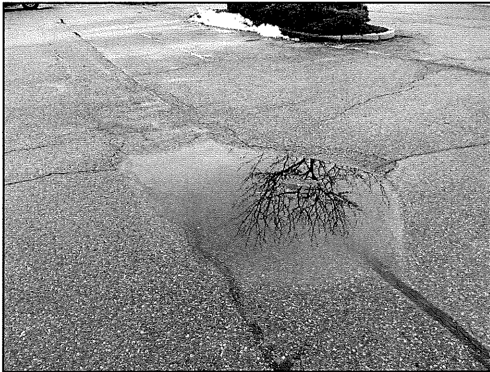
Photo 26: Puddling (see Photo Location Figure)
