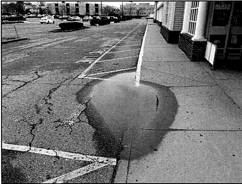
Photo 2: Puddling (see Photo Location Figure)
