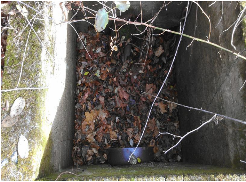
5) View of the concrete-constructed pit located on the northeastern portion of the Subject Property.
