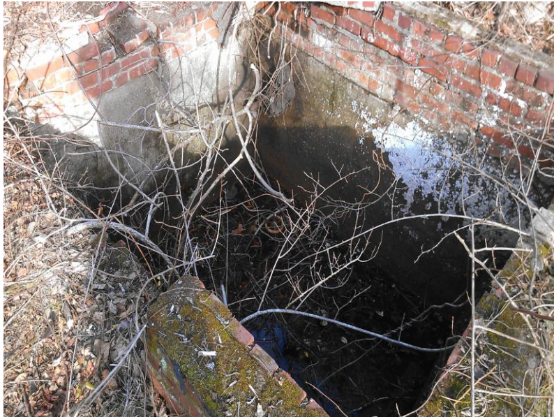
3) View of the brick-constructed pit located on the eastern portion of the Subject Property.
