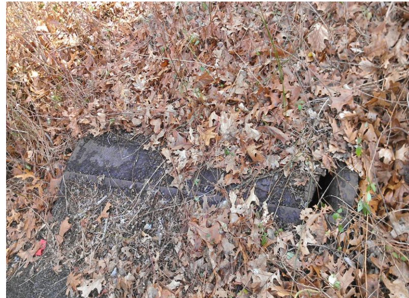
4) View of the partially exposed UST located on the eastern portion of the Subject Property.
