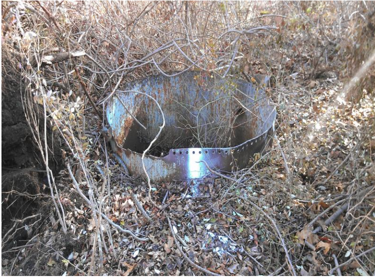
1) View of the metal cistern-like object located in the center of the Subject Property.
