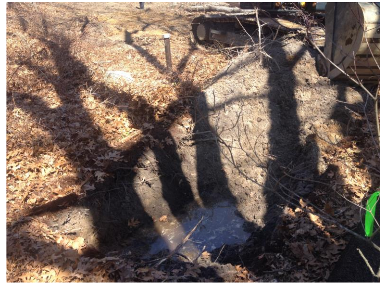
14) AOC-8: Acid Storage Tanks. View of test pitting activities in the vicinity of the Acid Storage Tanks.
