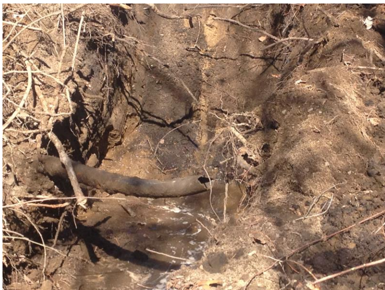
11) AOC-7: Waste Disposal Area No. 2. View of piping running through Waste Disposal Area No. 2.
