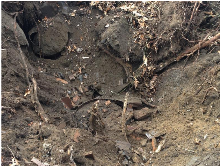
9) AOC-6: Drum Storage Area/Benzol House. View of debris in AOC-6 during excavation activities.
